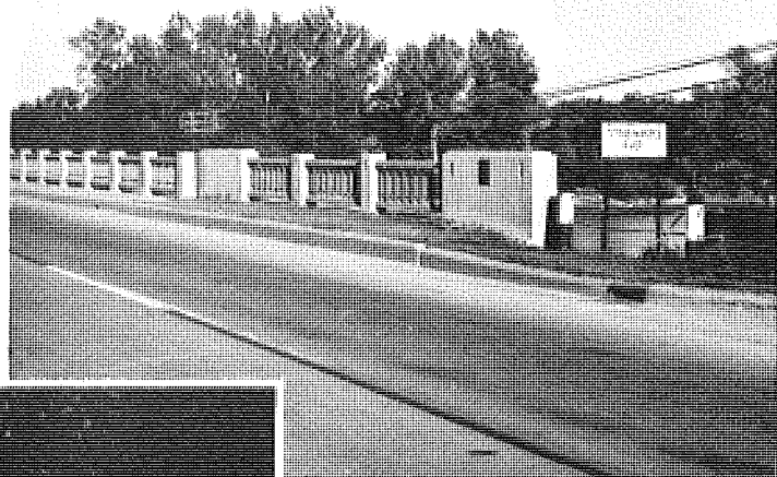
Figure 15. General view of bridge railing used on Michigan system after mid-1930's. Bridge is on M 46 west of Saginaw built in 1954. Note use of cable guardrail abutting bridge on right.
