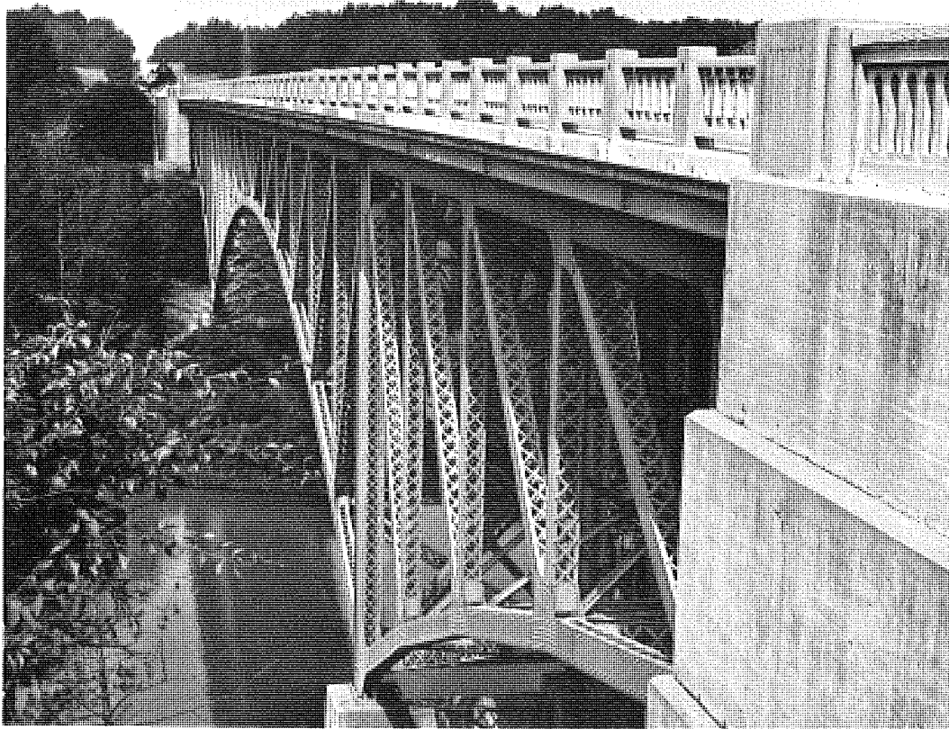
Figure 27. M 55 over the Pine River is a 3-span structure utilizing mostly latticed members that are difficult to paint. B03 of 51021 (Cooley Bridge) utilizes a design similar to that shown in Figure 22 (July 1972).
