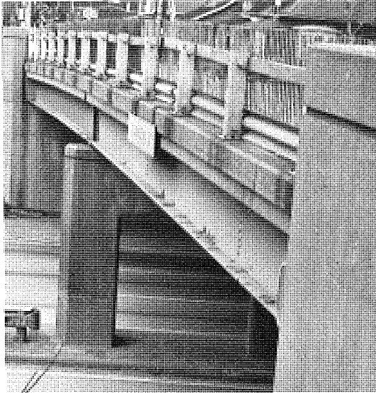
Figure 31. Top of lower flange of fascia beam shows blister and delamination failure 12 years after maintenance repainting. Note barricade at bridge railings while old painted rails are being galvanized (March 1974).
