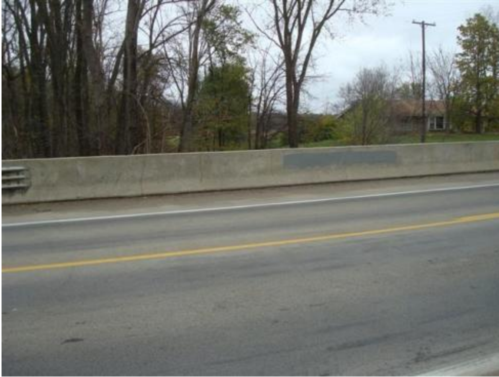
Figure 13. Vertical cracking in barrier wall, transverse cracking in the deck
