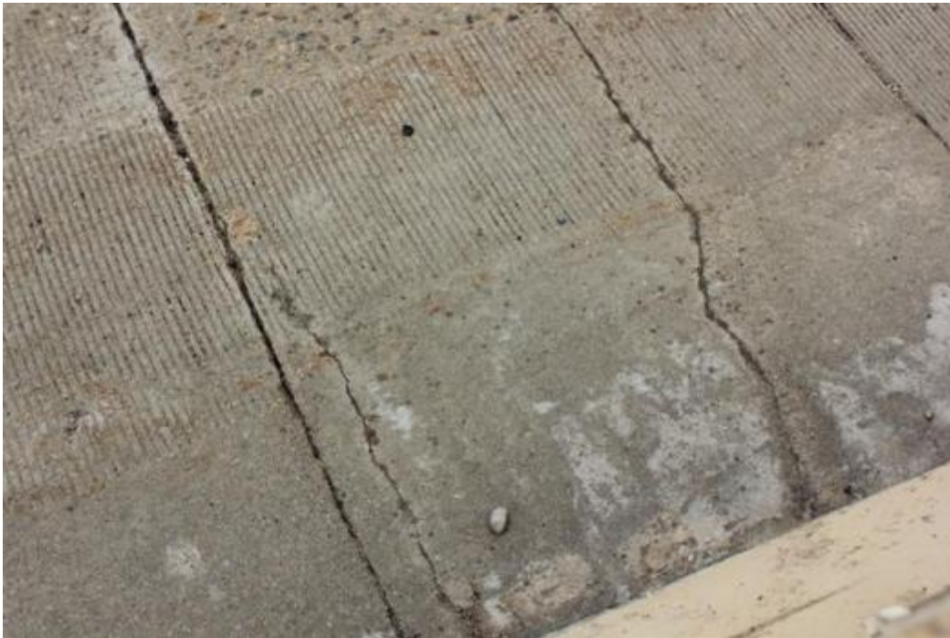
Figure 100. Close-up of transverse cracks
