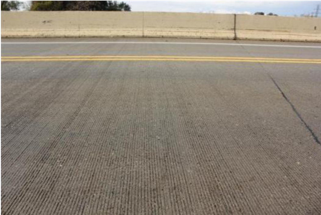
Figure 121. Transverse cracking at the pier area
