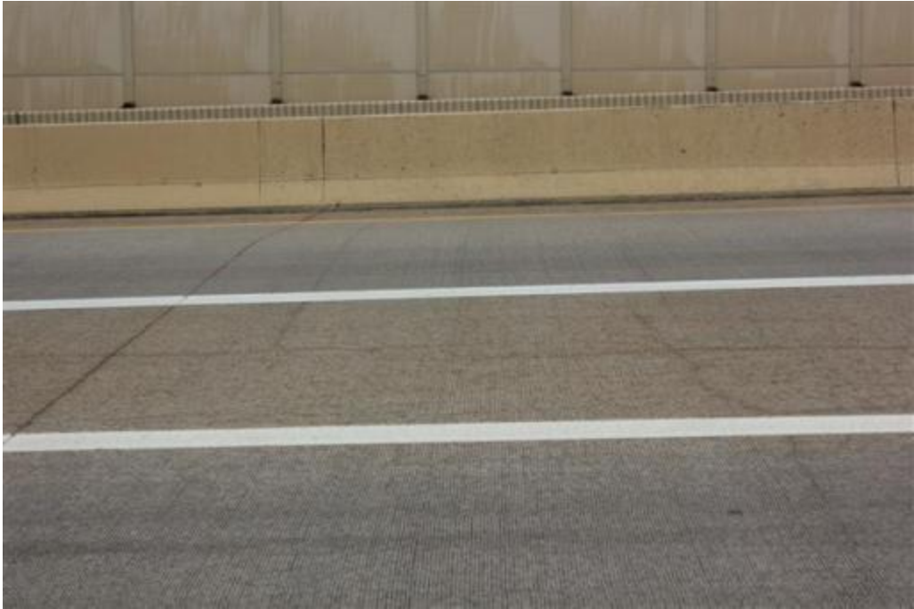
Figure 106. More transverse cracks in bridge deck
