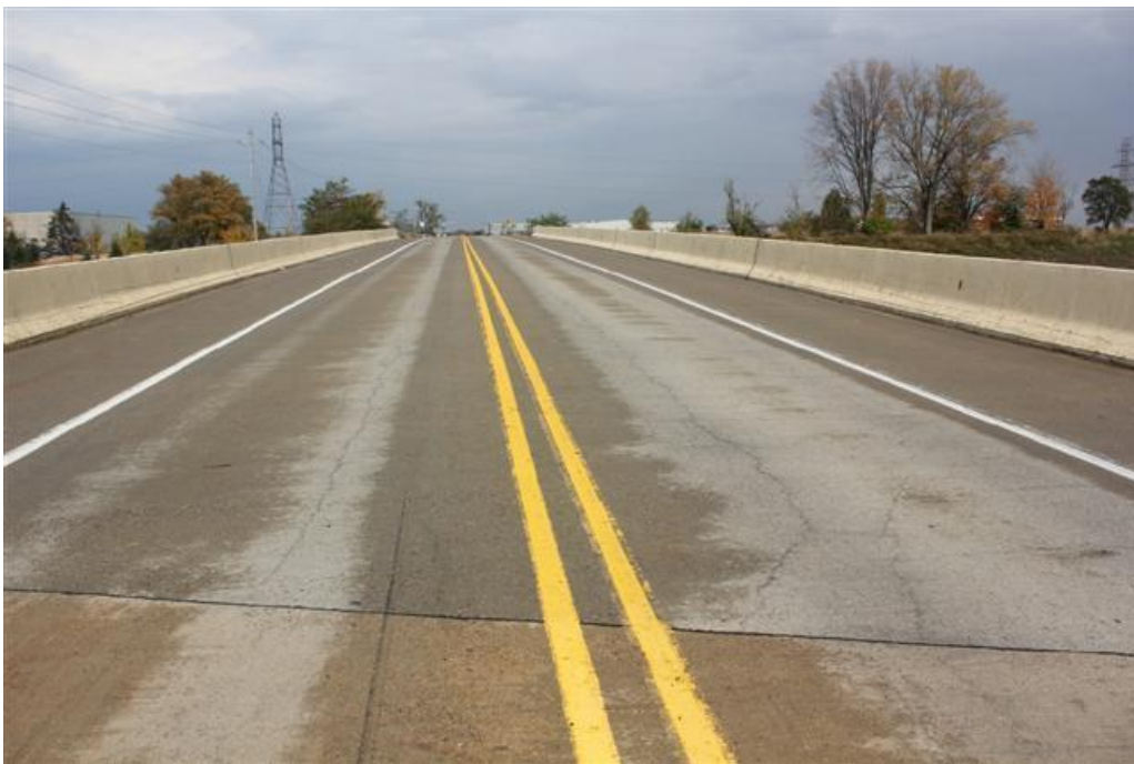
Figure 14. Typical longitudinal cracking (Bridge No. 11: Burlingame Rd. over M-6)
