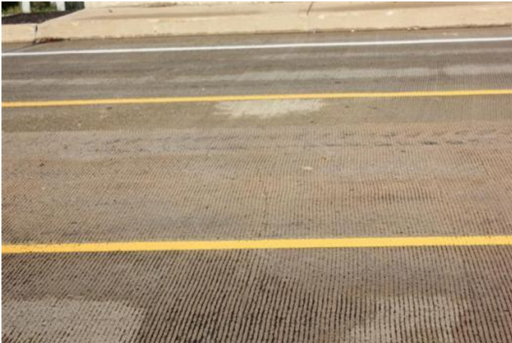
Figure 136. Transverse cracking in bridge deck
