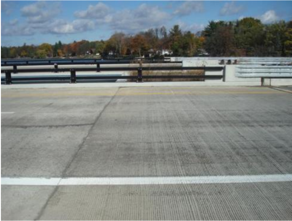
Figure 56. Longitudinal cracking in bridge deck
