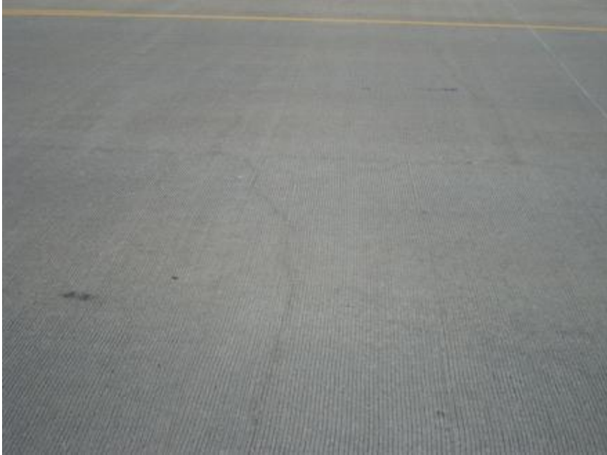
Figure 89. Transverse cracking in pier area
