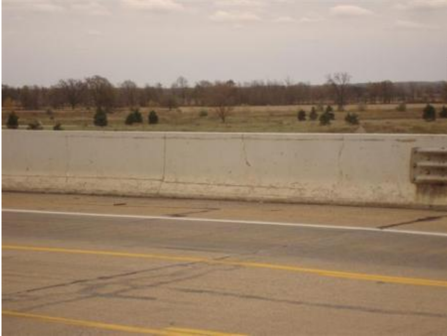
Figure 24. Cracking in barrier wall
