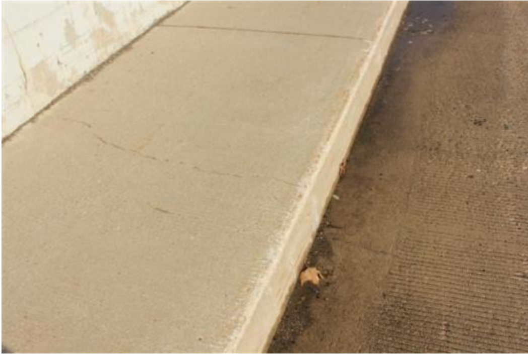
Figure 139. Transverse cracking in bridge deck and continuing into the sidewalk
