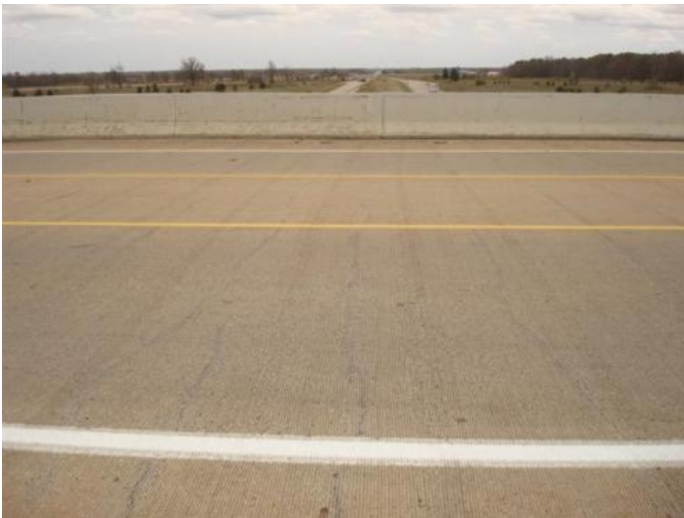
Figure 27. Transverse cracking in deck
