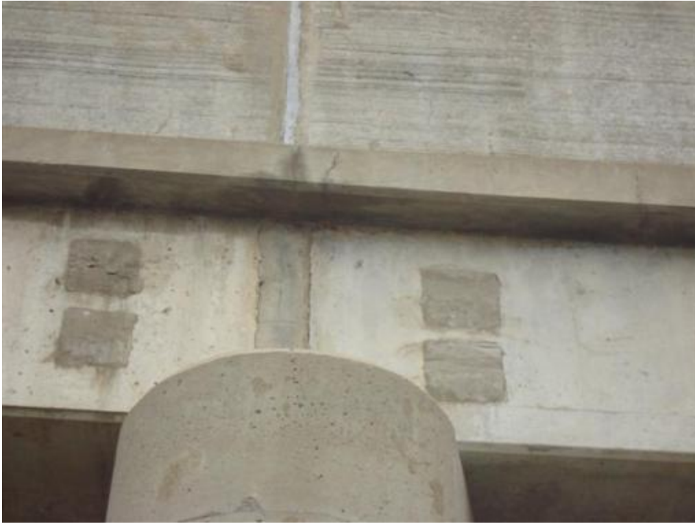
Figure 6. Transverse cracking in deck fascia
