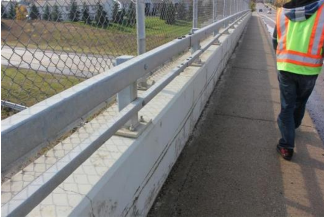
Figure 135. Cracking in barrier wall (typical)
