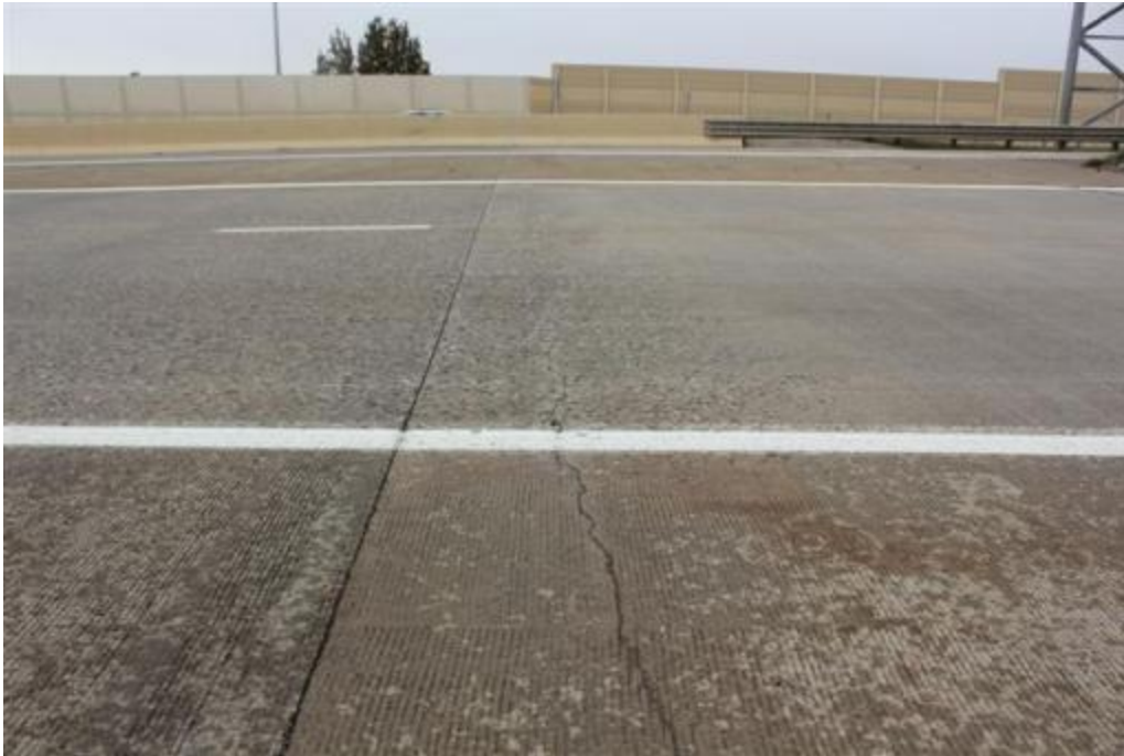
Figure 108. Large transverse crack at opposite abutment
