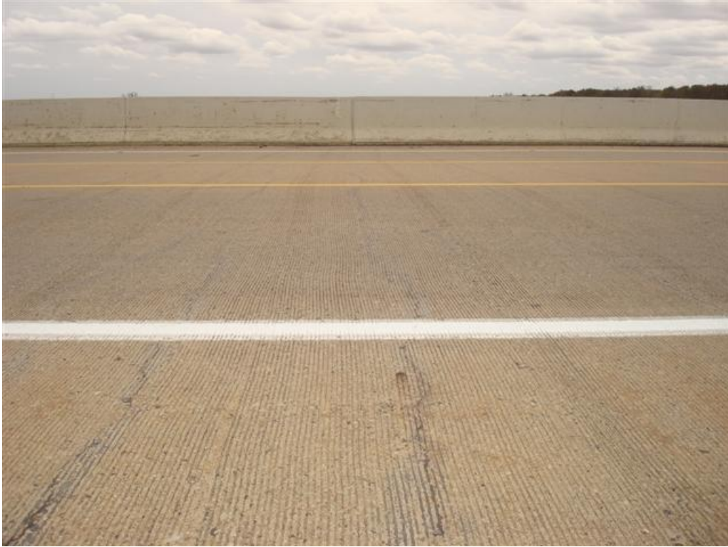
Figure 13. Typical transverse cracking in deck surface (Bridge No. 5: M-57 over US-127)
