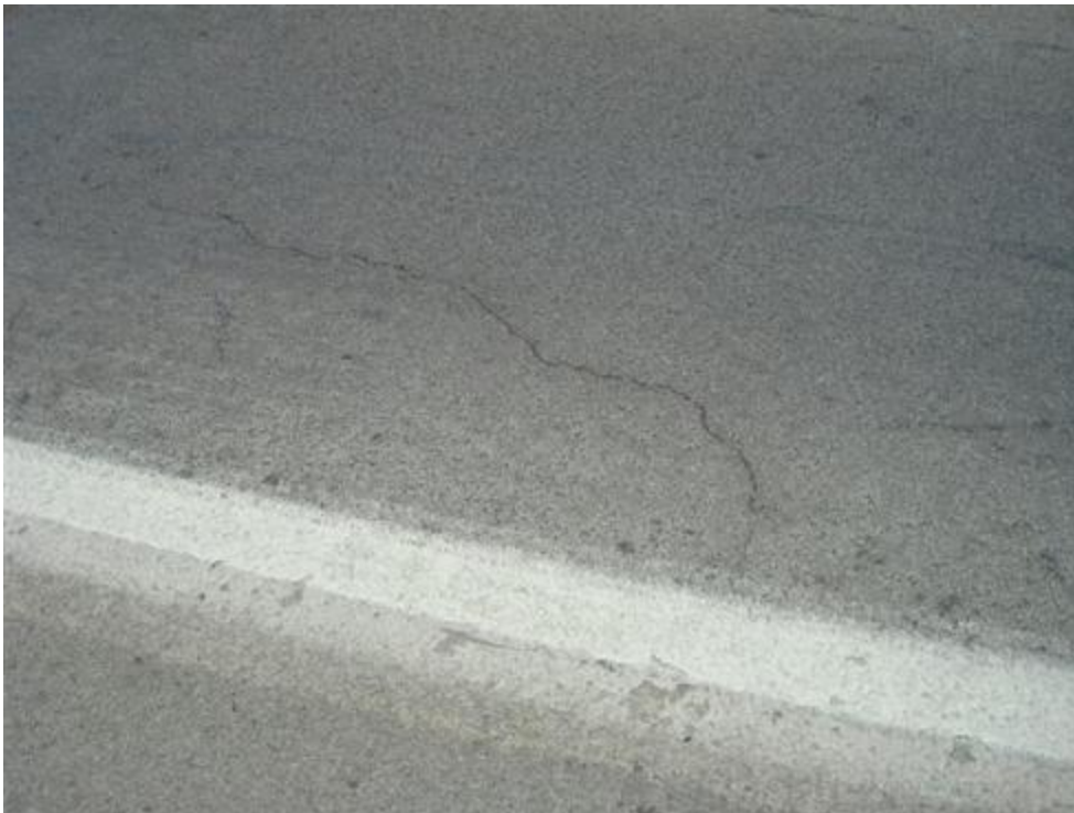
Figure 14. Longitudinal crack in the deck
