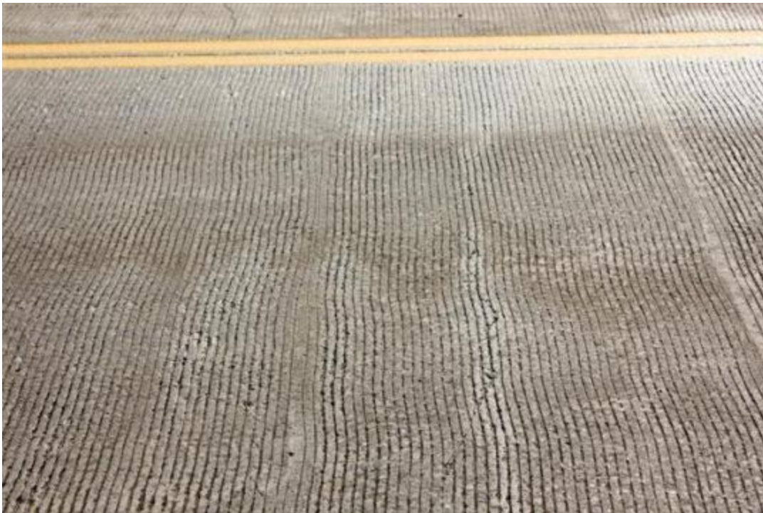
Figure 140. Evenly-spaced transverse cracks
