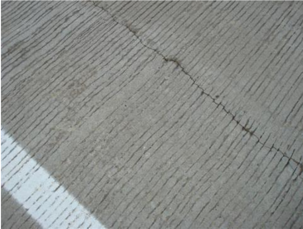
Figure 38. Close-up of longitudinal crack
