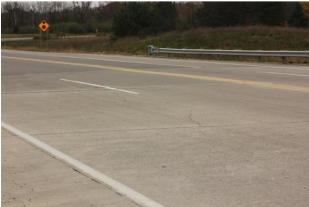
Figure 67. Longitudinal cracks in the deck
