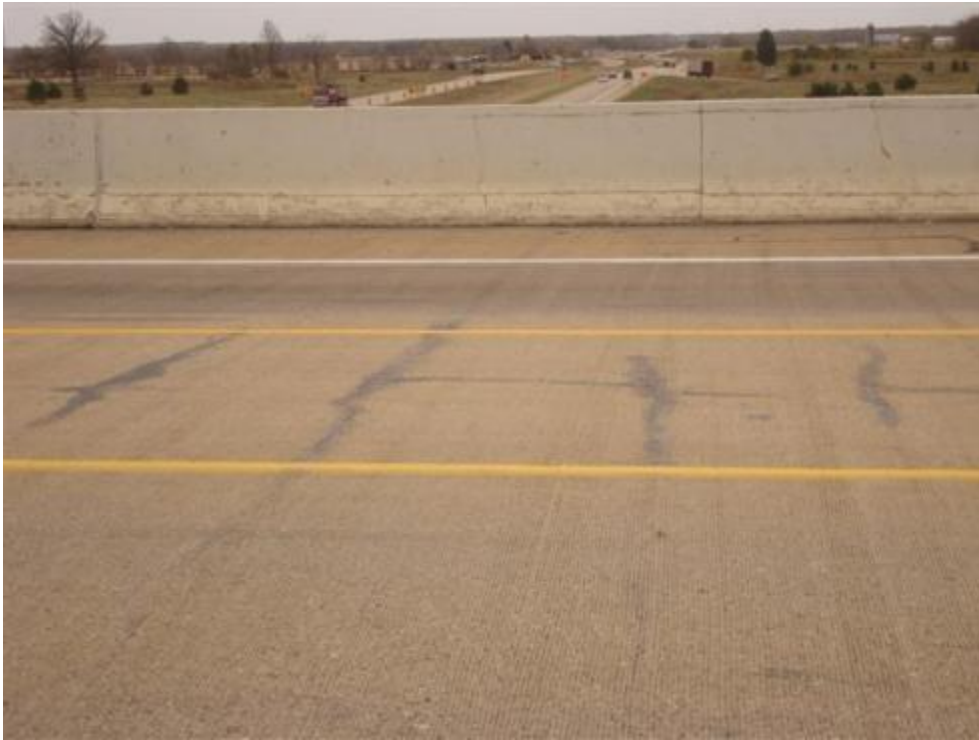
Figure 26. Transverse cracks in deck surface
