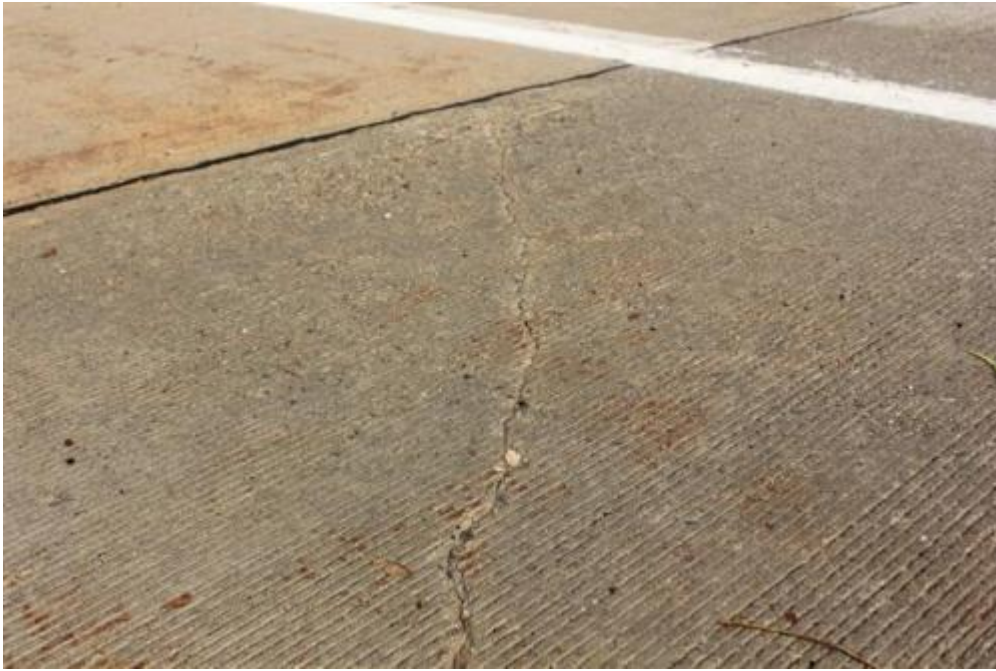
Figure 124. Diagonal cracking near the abutment
