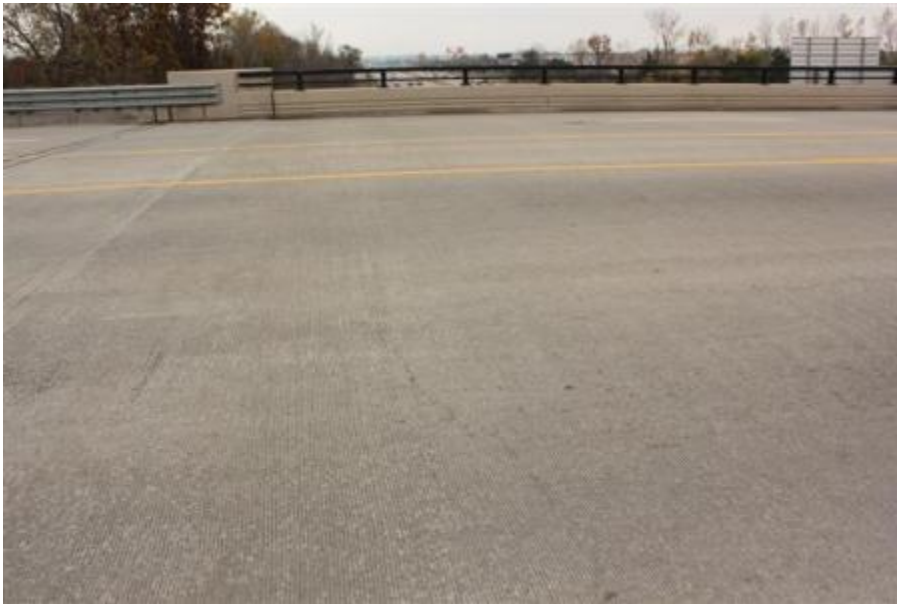
Figure 90. Transverse cracking in second span, near the abutment
