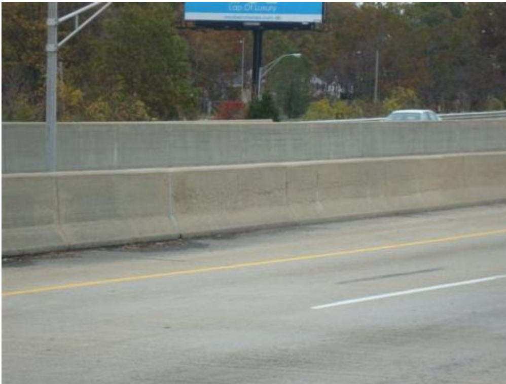
Figure 9. Extensive cracking in barrier wall
