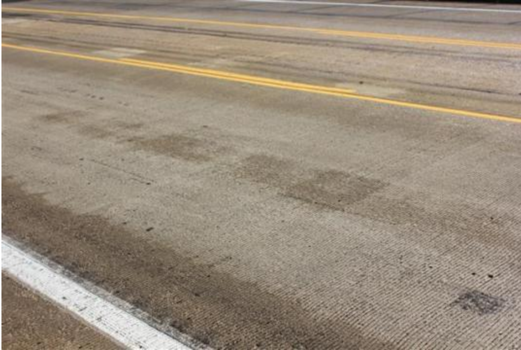
Figure 141. Random small longitudinal cracks
