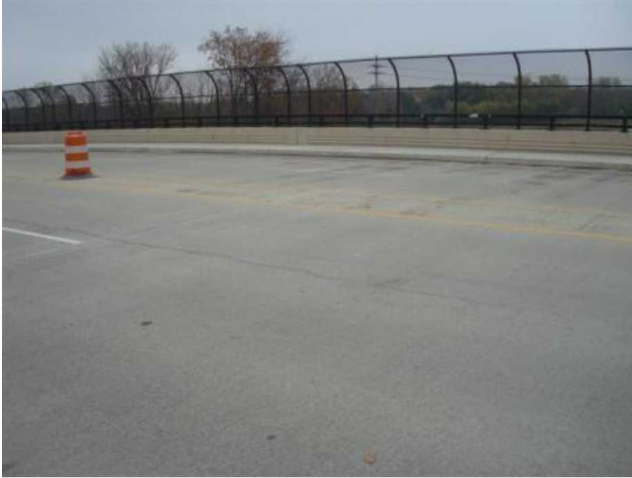
Figure 77. Large longitudinal crack in deck surface
