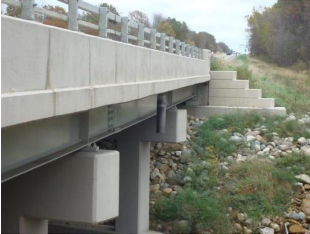
Figure 47. Cracking in barrier wall and deck fascia
