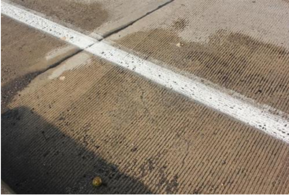
Figure 137. Longitudinal/diagonal cracking near the abutment
