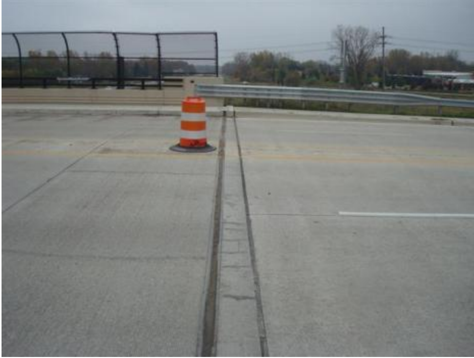
Figure 75. Longitudinal cracking in approach slab
