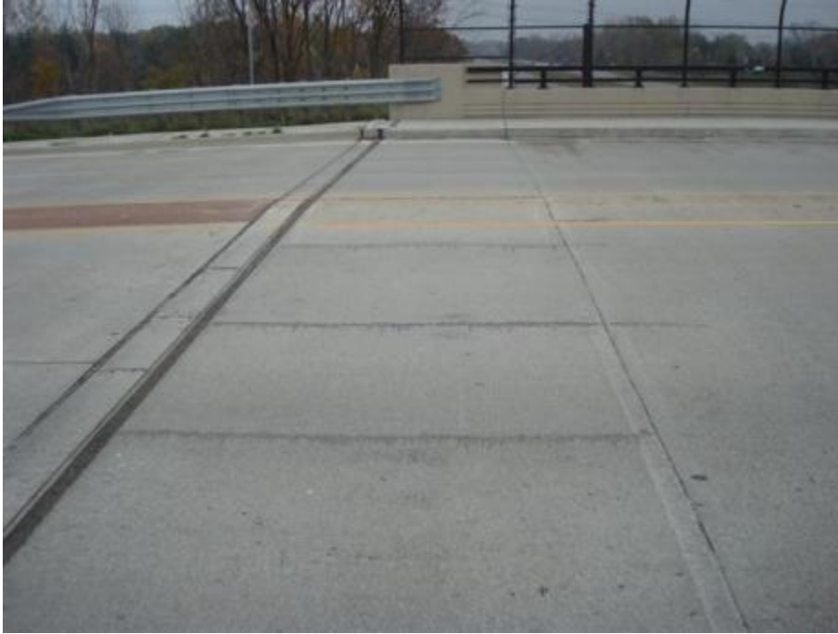
Figure 81. Almost identical cracking in opposite approach slab
