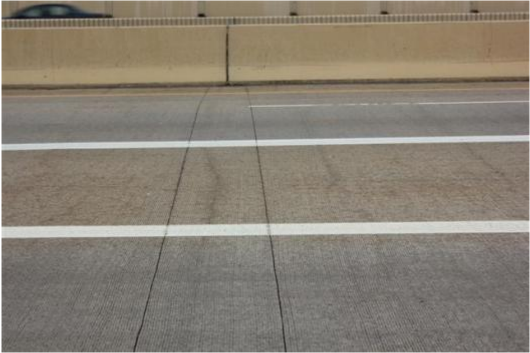
Figure 105. Extensive and evenly-spaced transverse cracks
