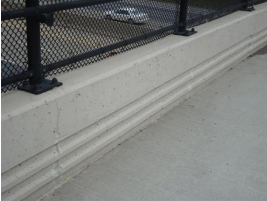
Figure 86. Cracking in barrier wall (typical)
