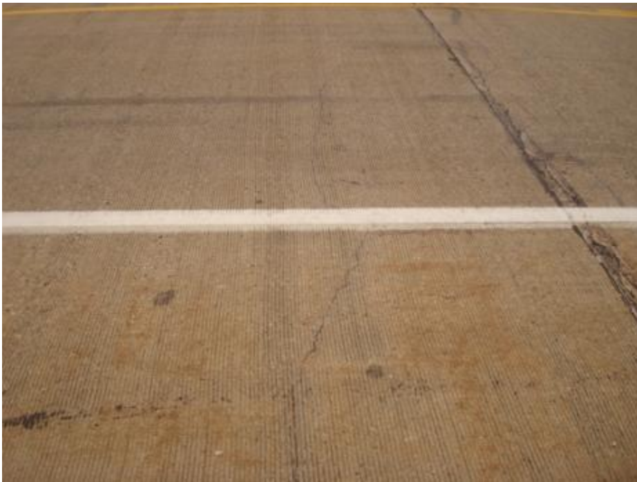
Figure 25. Transverse crack near construction joint
