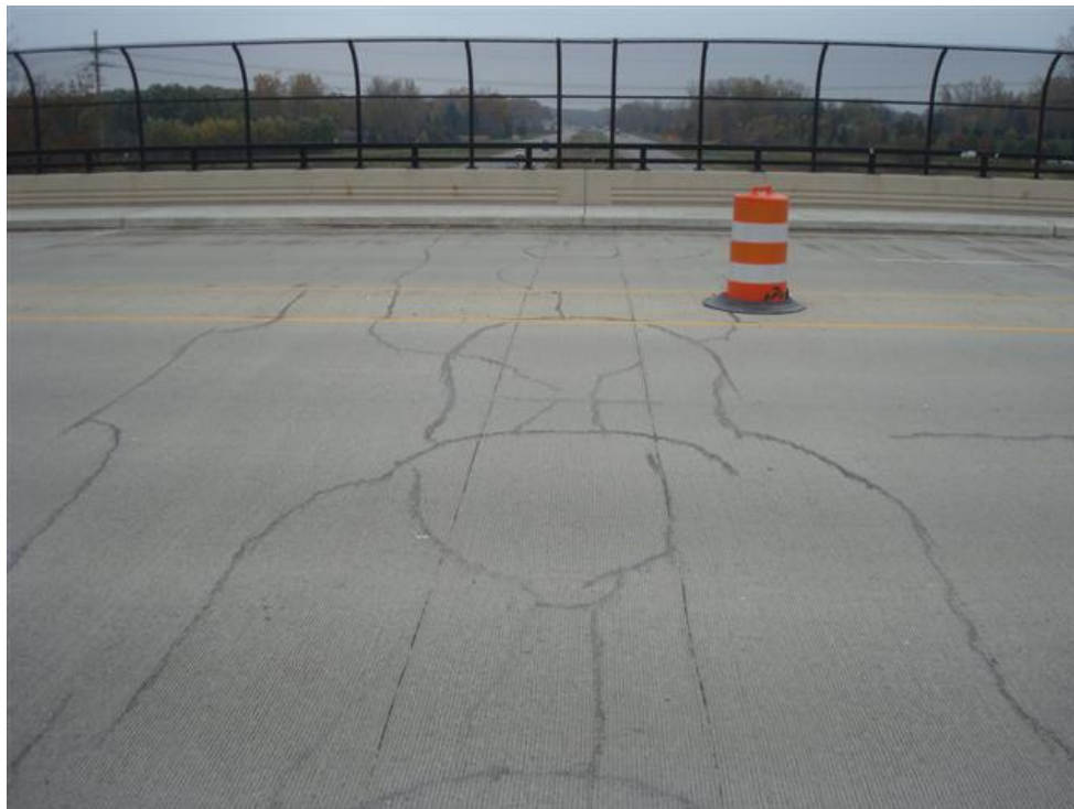
Figure 12. Transverse cracking over pier/negative moment region (Bridge No. 13, 26 mile Rd. over M-53)
