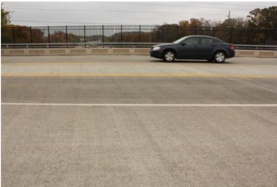
Figure 93. Possible longitudinal crack in the middle (it was not clear in the investigation whether it was a crack or roughed surface)
