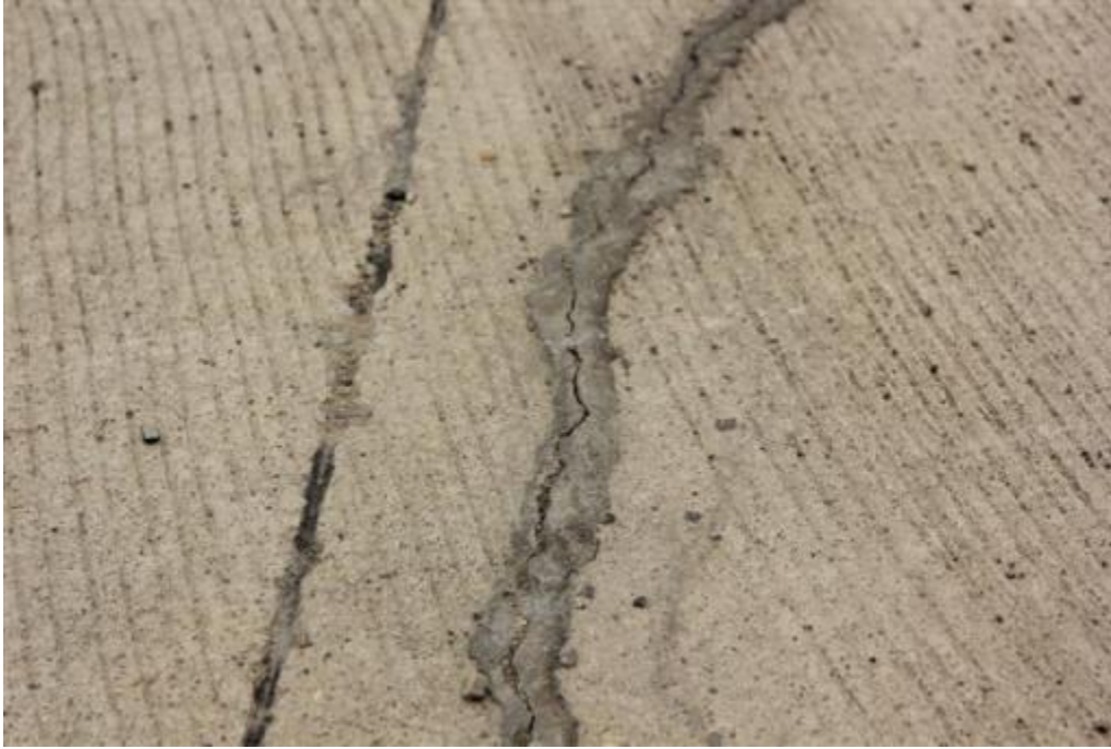
Figure 66. Close-up of transverse crack (note how it cracked through the repair)
