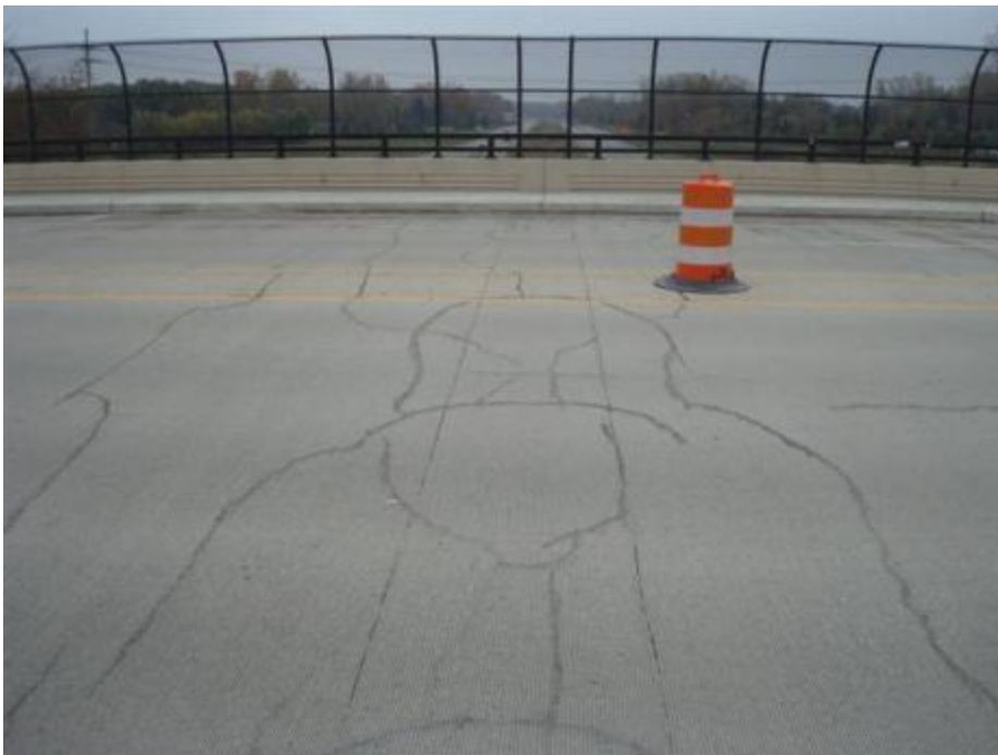
Figure 78. Heavy transverse cracking in pier area
