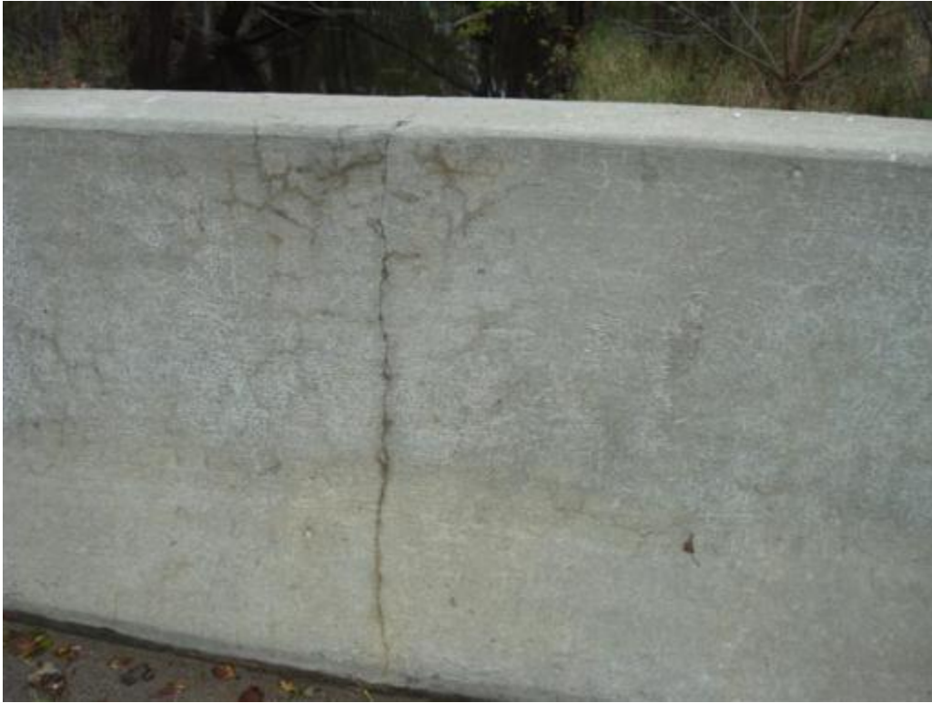
Figure 17. Large crack in barrier wall
