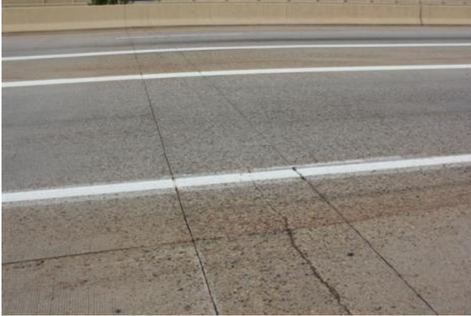
Figure 99. Transverse cracking bridge deck, near the abutment
