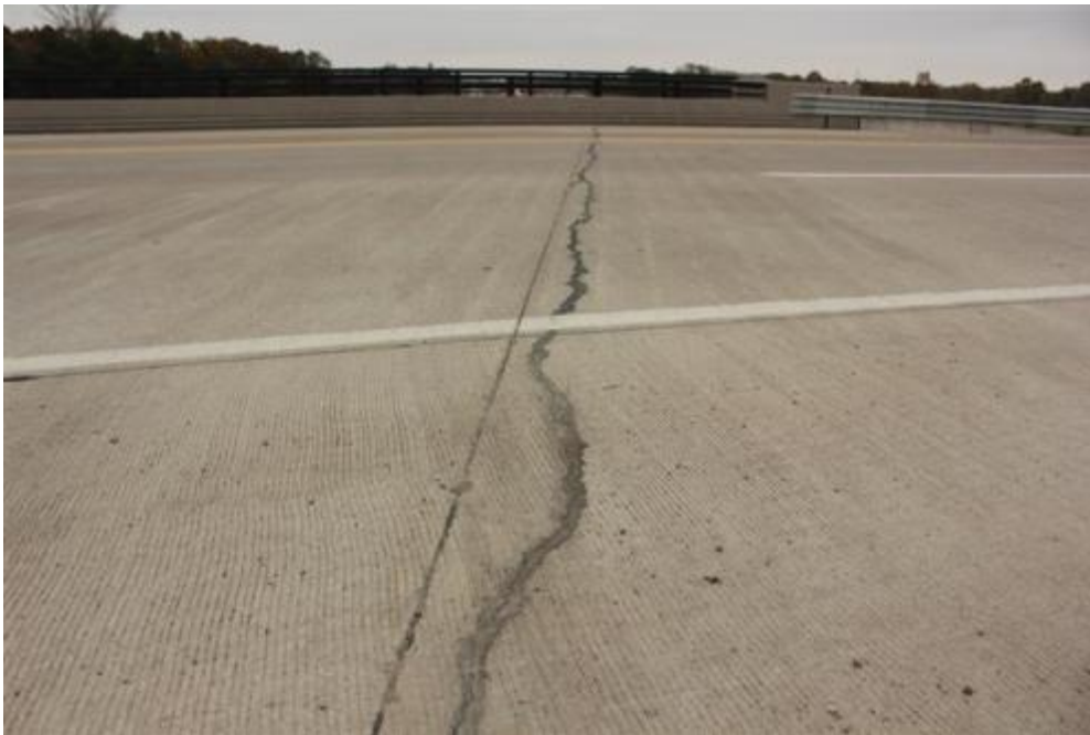
Figure 65. Large transverse crack at the abutment
