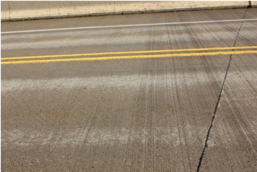
Figure 127. Evenly-spaced longitudinal cracks
