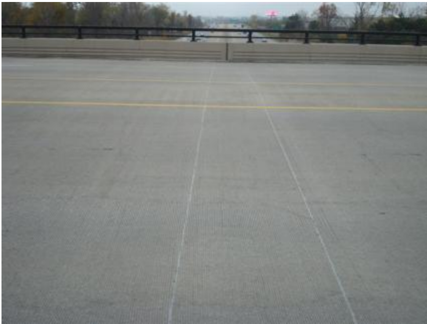
Figure 88. Longitudinal and transverse cracks in pier area
