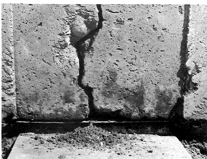
The joint crack after removal of soil material near the slab edge.
