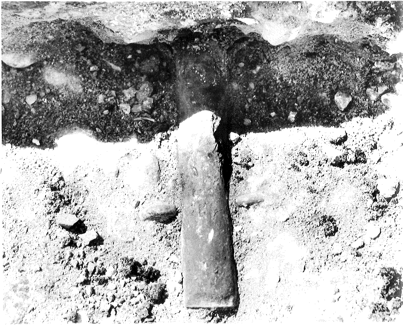
Figure 12. Corroded dowel in place in 9-year-old pavement. Sta 496+25, Proj 72-7, C5; constr 1948 (May '57).
