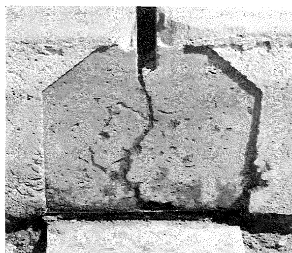
When this excess soil was removed, additional compacted soil was found in the joint crack.
