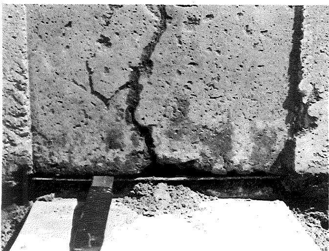
The base plate was found to be depressed, and the space between the plate and slab filled with fine soil.
