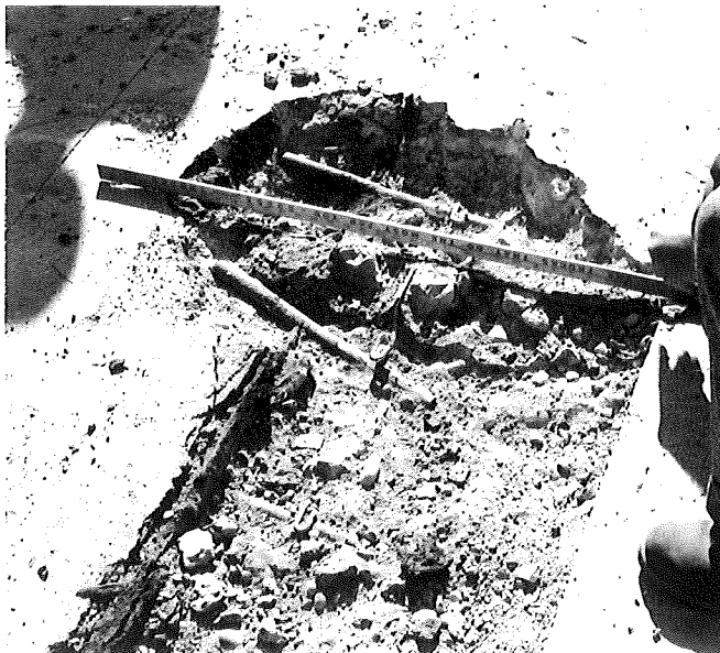
▲ Figure 9. Dowel misalignment during concrete placement, due to inability of assembly to hold dowels in place. Sta 56+27, Proj 63-67, C4; constr 1947 (Oct '52)
