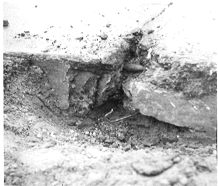
▲ Figure 10. Blow-up at joint with dowels and bar assembly too close to surface. Sta 297+22, Proj 72-7, C5; constr 1947 (Nov '54)
