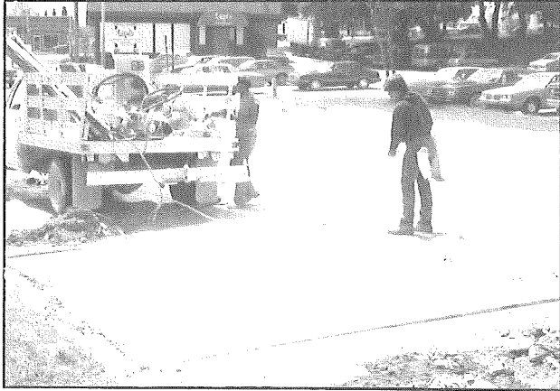
Figure 26b. The joint grooves are cleaned by sand blasting and compressed air prior to sealing.
