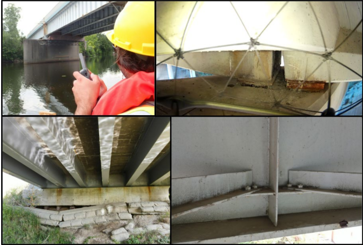
Figure 3.2.28: Example situations highlighting the utility of drones in surveying locations that are otherwise difficult to assess. A drone pilot captures imagery of bridge beams under I-96 at Grand River (top-left), a caged drone system is able to get very close to difficult to see areas (top-right), imagery of bridge substructure at Beyer Rd (bottom-left and bottom-right).
