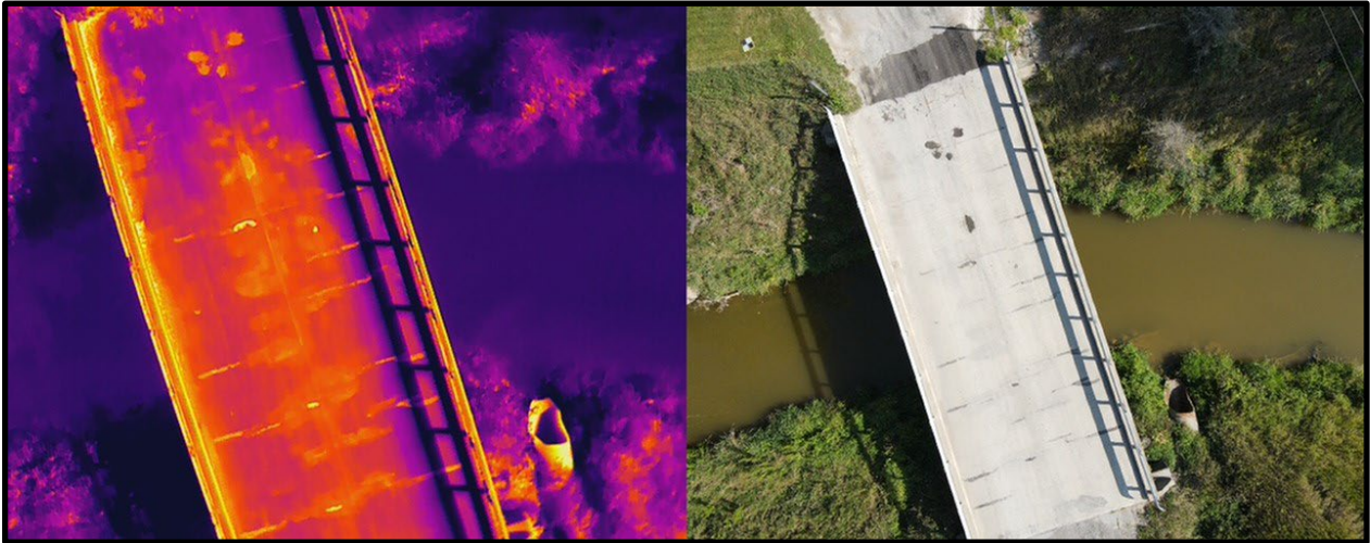
Figure 3.2.1: Beyer Road bridge, near Saginaw, MI, showing thermal data (left) and optical data (right) from the August 17, 2021 data collection. We are recommending this low-traffic bridge with known defects and two years of UAS data as an excellent location for the planned spring 2022 UAS-assisted bridge inspection demonstration day to be held with MDOT bridge inspection staff. (move this to body of report, shouldn't be under figure title)
