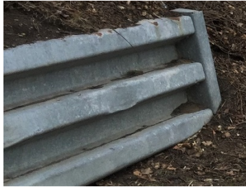
Steel Bin Wall
