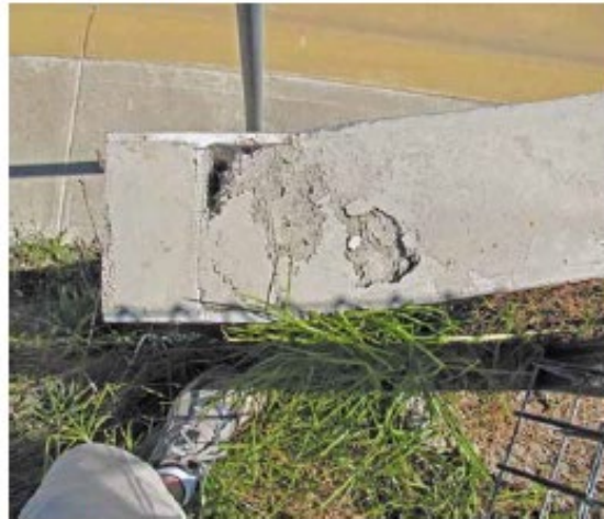
Incomplete filling of concrete around supporting steel posts with potential for water penetration and corrosion
