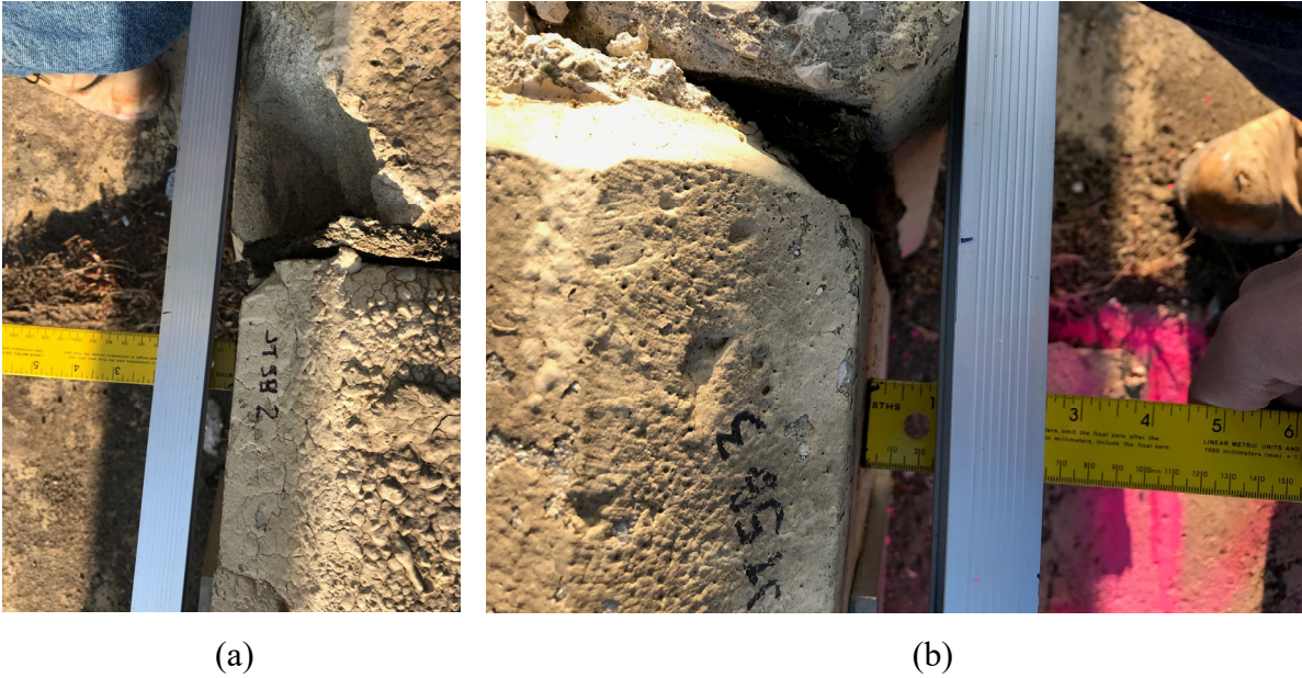
Figure B.1. Manually measured movement of the M-10 wall panel at the top wall parapet in January 2020.
