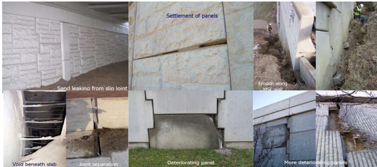
Figure 1.9. Observed problems in MSE walls (Narsavage 2006)
