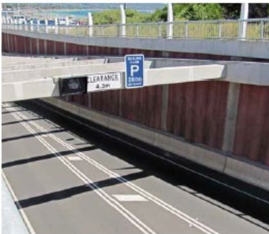
Exposed bored pile retaining wall in sound condition with no evidence of significant cracking, movement, water penetration or corrosion.
