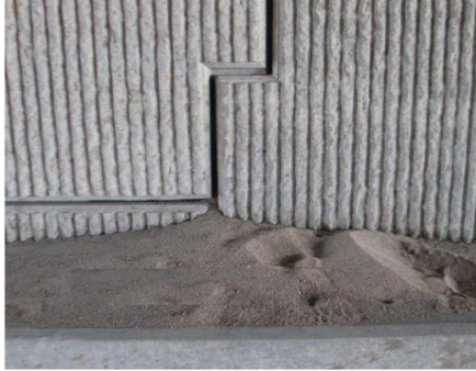
Loss of Backfill
