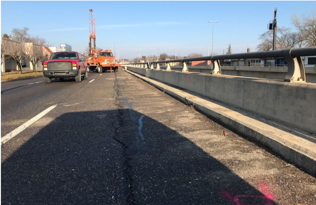
Figure B.2. Top road surface at the top of the suspected failed M-10 wall panel (January 2020); major tensile crack in asphalt surface evident parallel to wall face.
