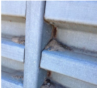
Steel Bin Wall
