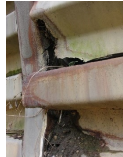
Steel Bin Wall
