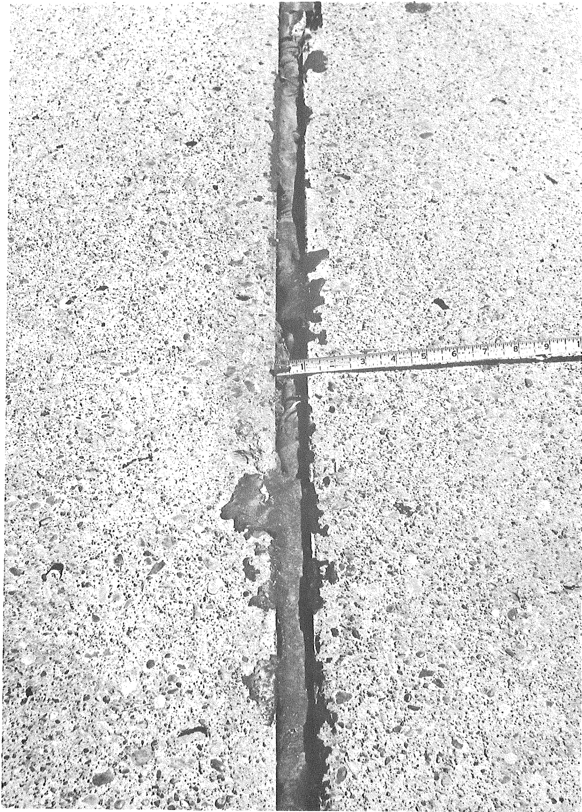
Figure 3. Typical joint width and sealant condition.
