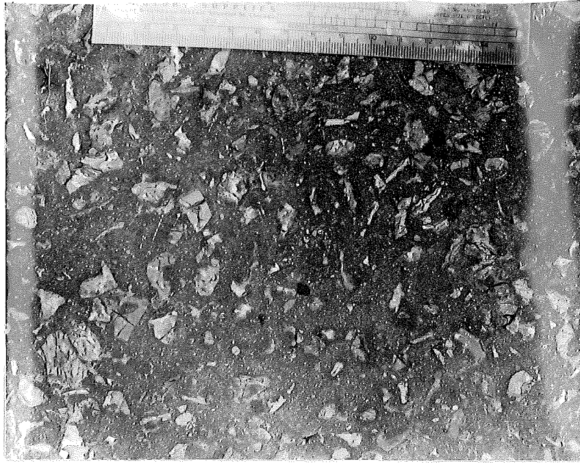
Figure 12. Condition of Surface of Recsp on US-10 north of Flint, Conct. Project P 25-4, C11, taken 2-23-49. Wallace Limestone.
