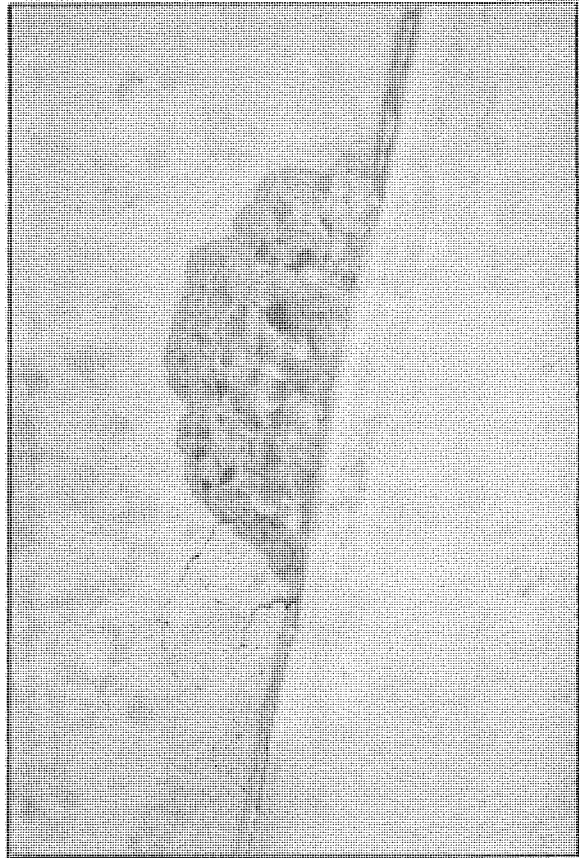
Figure 6. Surface spall (about 6 in. long).
