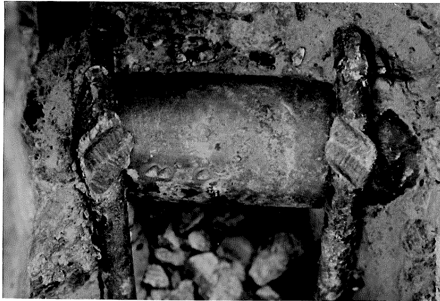
Figure 3. Typical surface condition of nickel clad dowels.
