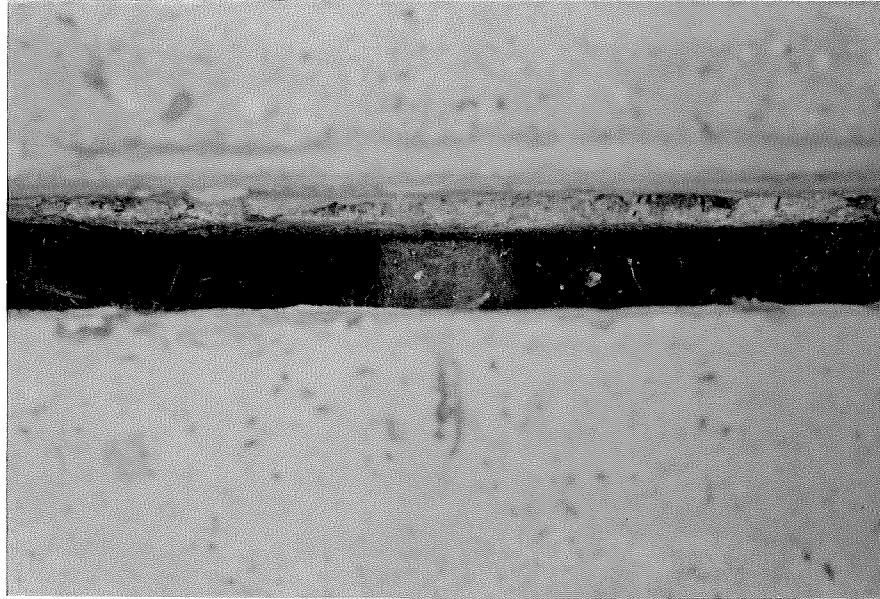
Figure 5. Typical corrosive condition of chromium-steel dowels.
