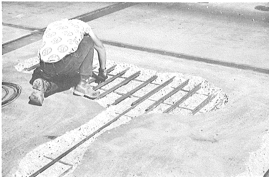
Figure 2 (left). Deck repair of spalls over bar splices, where cover was 1-1/2 to 2 in. (X01 of 38101).
