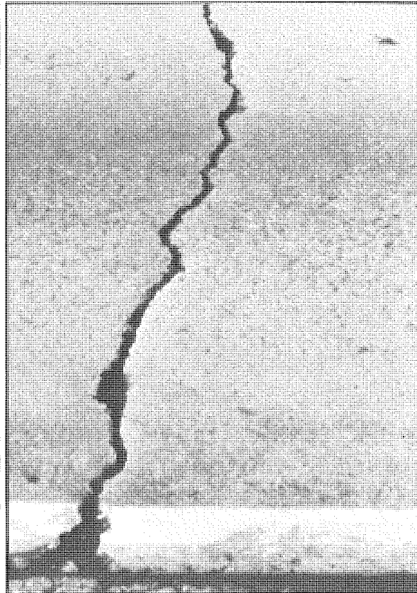
Figure 6A. Transverse crack with reinforcement intact.
