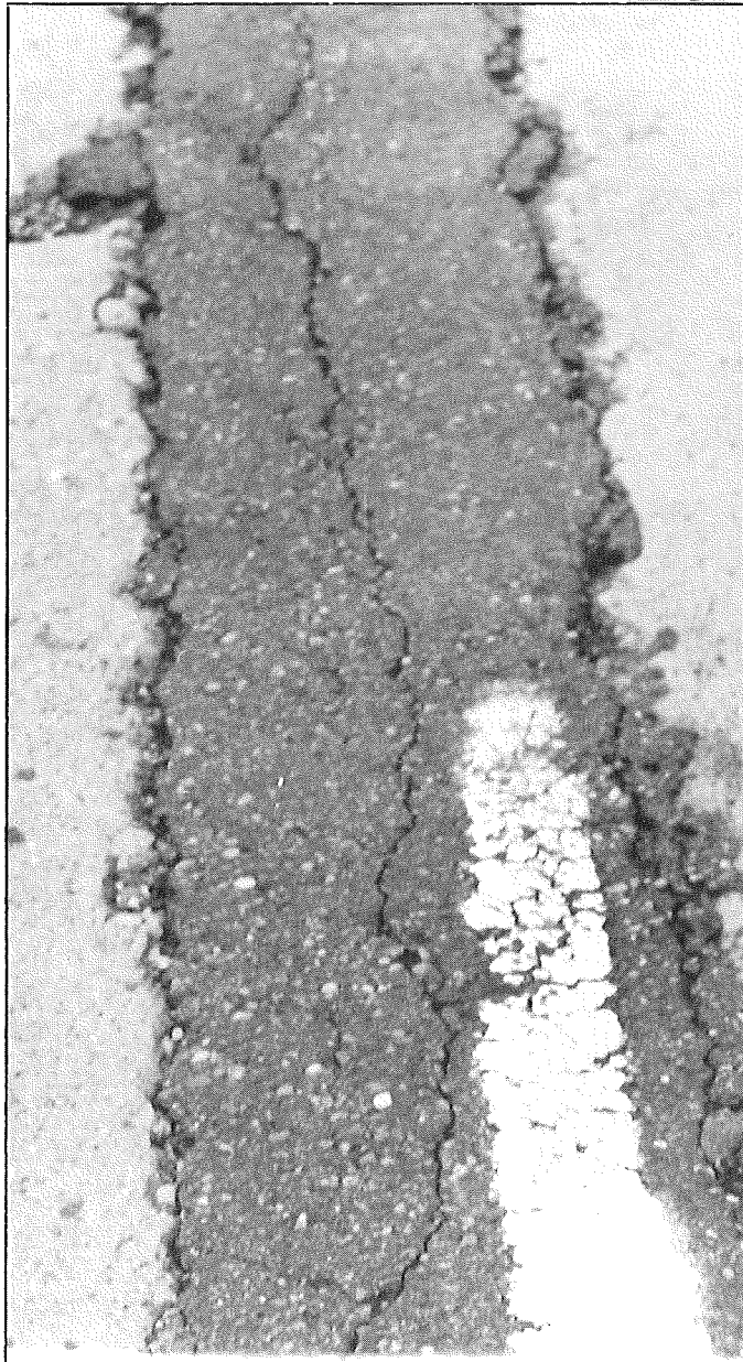
Figure 23. Ravelling along edges and cracking over plane-of-weakness crack.
