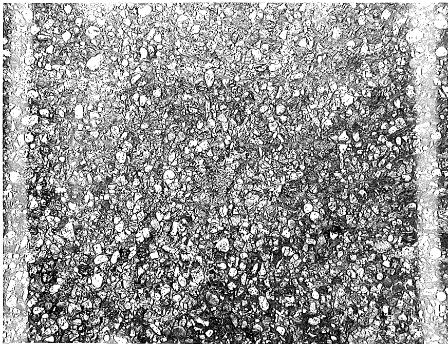
B. View of surface showing typical condition of aggregate. Resealed Wallace stone in 1940 (from Maintenance Engr.) State Reward 4145 1920 M-47 2 miles So. of M-46, So. 1 Mile.
