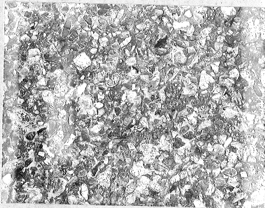
B. View of surface showing typical condition of aggregate Wallace stone 26A modified R-25-4, 011, 1948, US-10 Dort Highway Flint just No. of Carpenter Rd., Center two lanes of a four lane highway.
