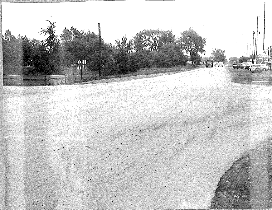
A. Typical condition of surface. No pitting. Shows signs of slight abrasion due to material brought onto intersection by traffic.
