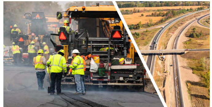
Using two pavers in close formation was found to be an important strategy for increasing the durability of asphalt roads.
