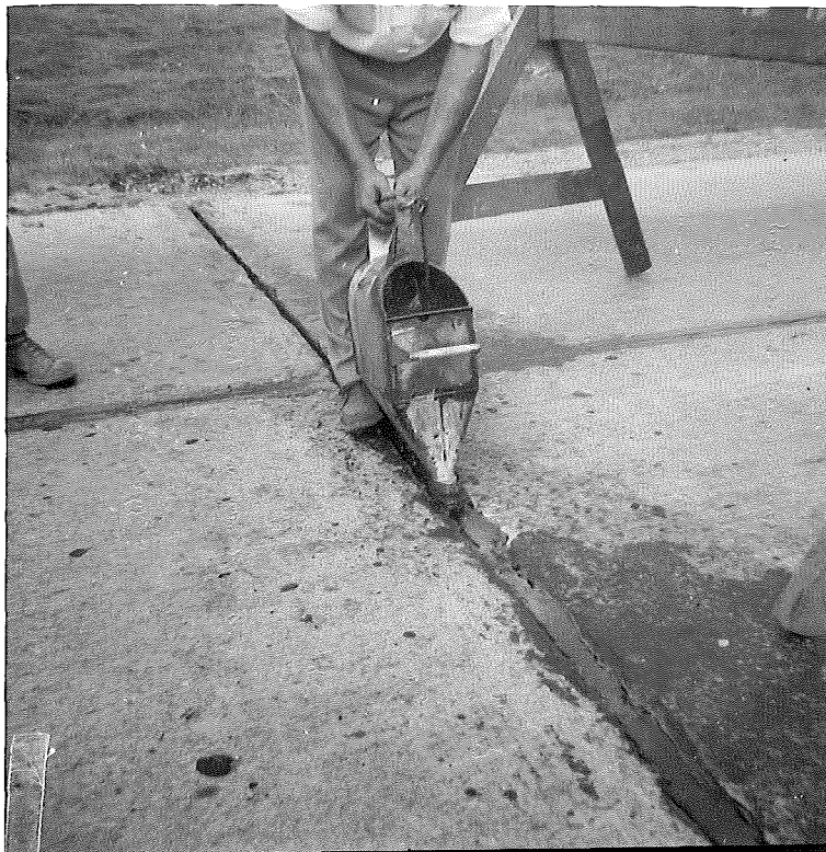
11. Pouring new matl. into pre- viously cleaned expan. joint. US16 near Lan- sing airport. BRD--8-18-47
