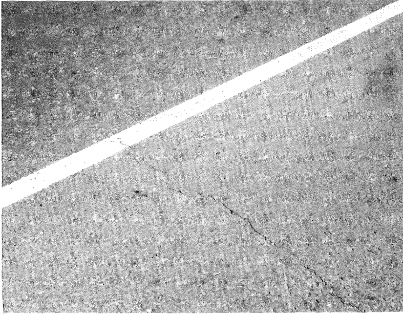
Figure 9. Right-angle reflection cracking in non-reinforced resurfacing, over intersecting transverse and longitudinal joints in the old base concrete pavement, after eight months service (May 1956).
