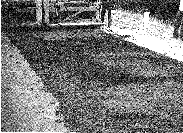
Extreme buckling of reinforcing steel behind the paver, protruding through binder course.
