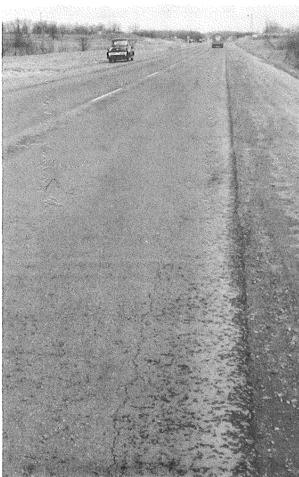
Figure 10. Reflection crack in non-reinforced resurfacing over longitudinal construction joint between old base pavement and 2-ft widening strip (April 1956).
