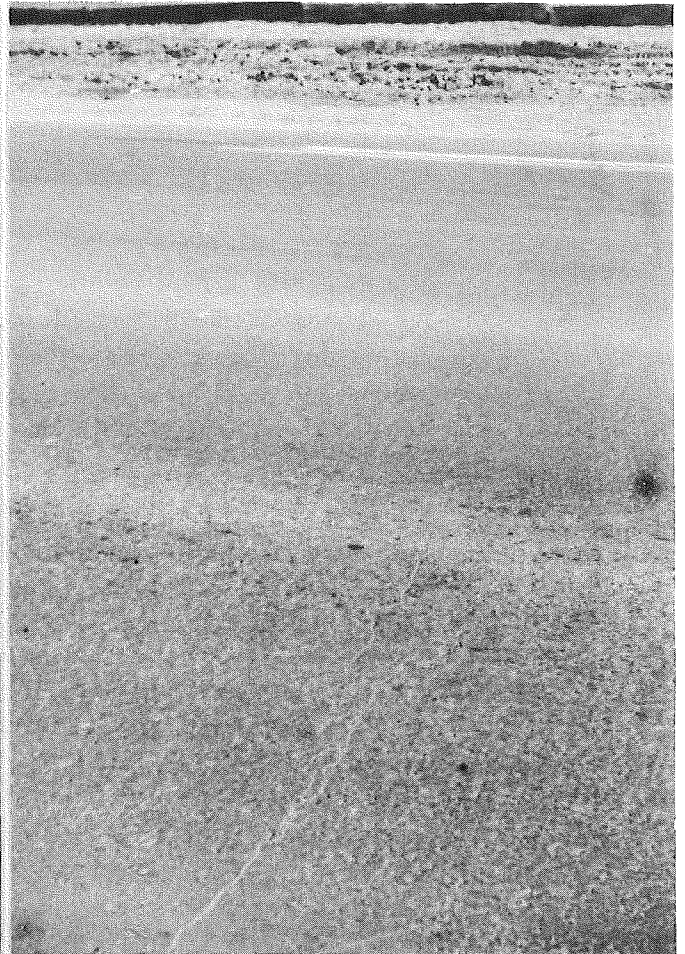
Figure 11. Reflection crack in continuously reinforced resurfacing section, showing staggered pattern of leading edges of adjacent mesh sheets (turn-off lane for US 23 at far edge). (May 1956)
