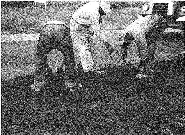
Wire cutting at edge of an area of buckled steel.
