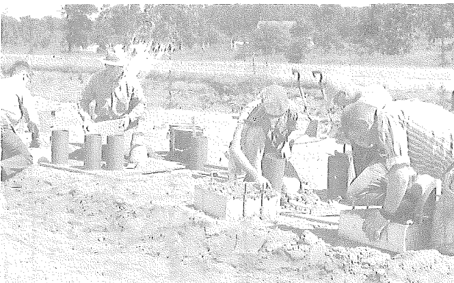
Figure 11. Three Compression Test Cylinders Were Molded From Each of the Three Samples in the Batch.
