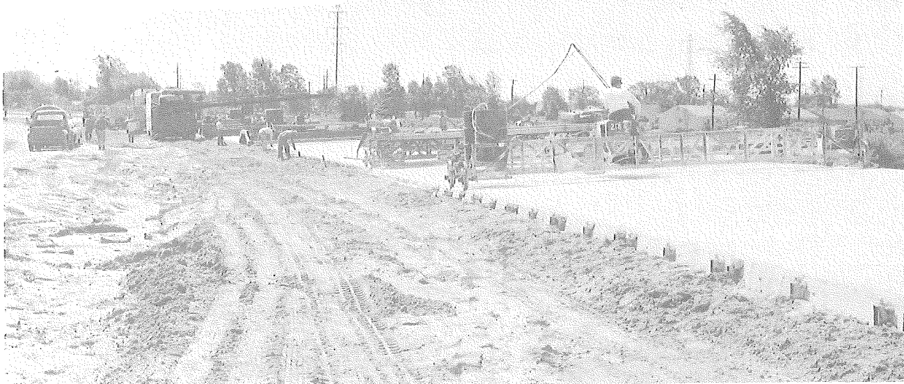
▼ Figure 21. The Curing Compound Spreader Brings Up the Rear of the Paving Train.
