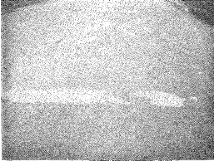
WB M-142 in Pigeon, Huron Co. Approximately 50% of the thermoplastic material remains intact. The pavement surface is not in good condition.
