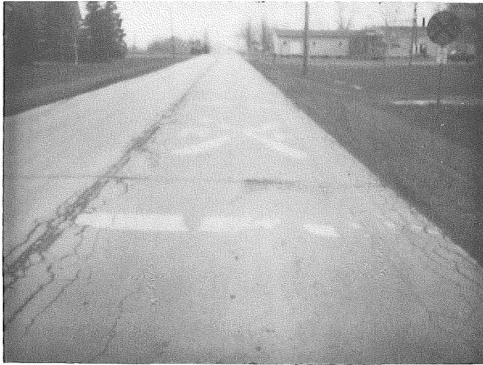
WB M-25 in Unionville, Tuscola Co. Approximately 40% of the thermoplastic marking has disappeared after one winter. Note rough pavement surface.
