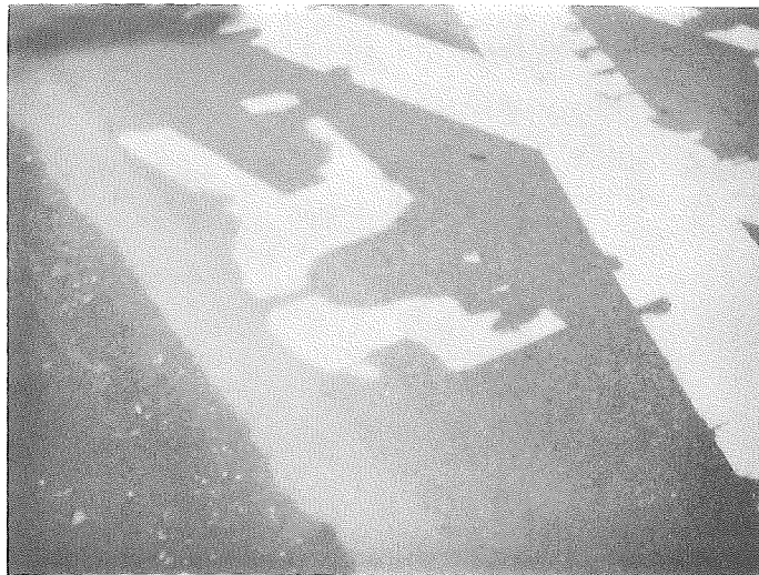
Considerable chipping has taken place with a good pavement surface. This could be the result of poor adhesion or snow plowing.
