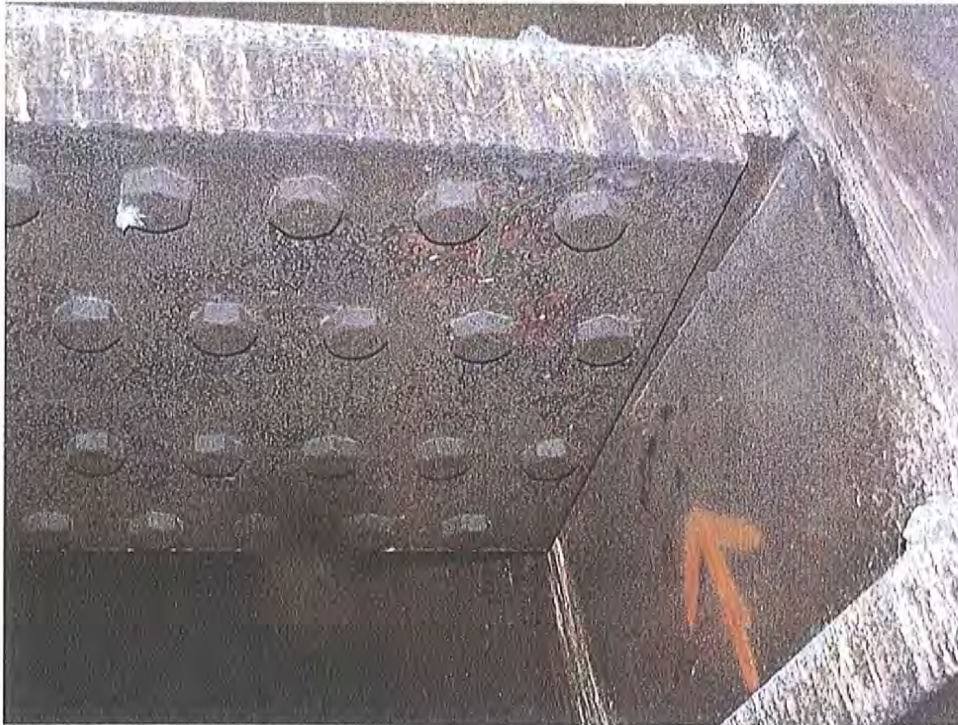
Figure 5 - Bolted field splices connect the girders to the pier cap. Crack in the face of the bottom fillet weld
