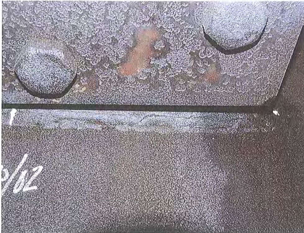
Figure 12 - Crack in the face/toe of the bottom fillet weld
