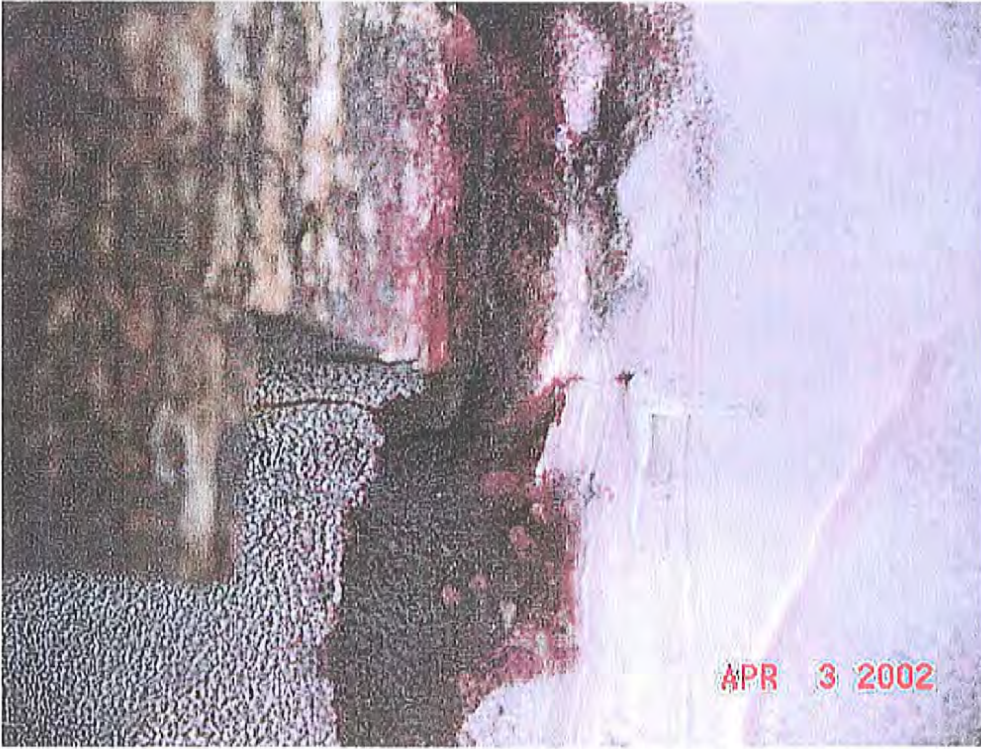
Figure 9 - Dye penetrant applied to the crack area in the web
