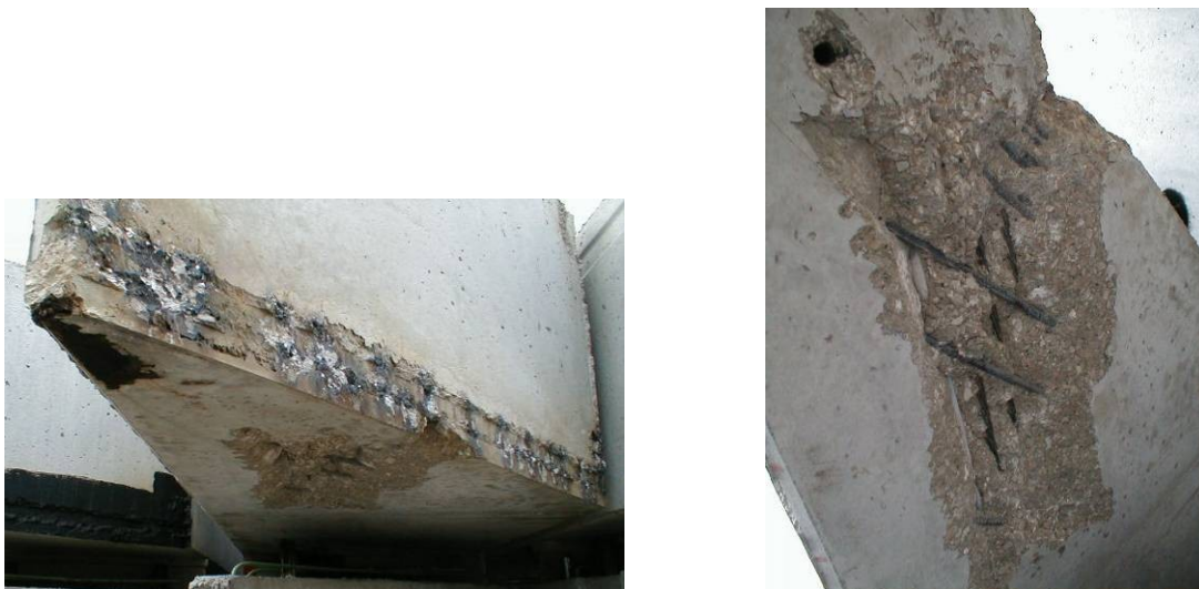
Figure 1 End Damage of Pre-tensioned Box Girder
