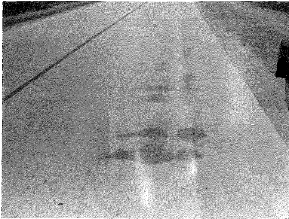
Figure 7. Discoloration in north lane, Station 85+40. Concrete not cracked or checked in dark areas.
