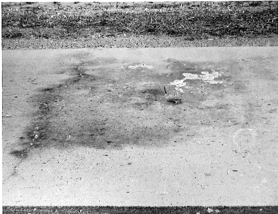
Figure 4. Appearance of pavement between Station 88+20 to 88+25. Concrete discolored and scaled in north lane only. Cracking extended across entire pavement.
