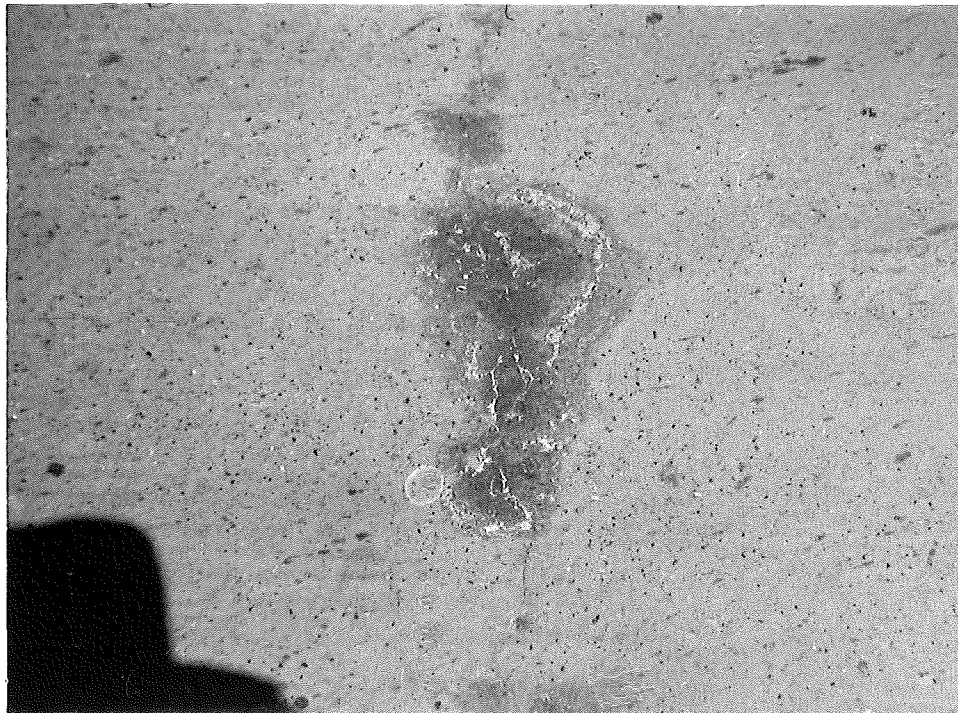
Figure 6. Excretion of white material in localized areas. Station 88+05.
