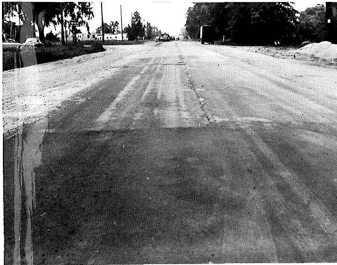
FIGURE 8. SHOWING POINT OF DIVISION BETWEEN BITUMINOUS BREAKER STRIP AND AE-3 AND SAND. STATION 249+46 LOOKING SOUTH FROM ABOUT STATION 250. JUNE 13, 1952
