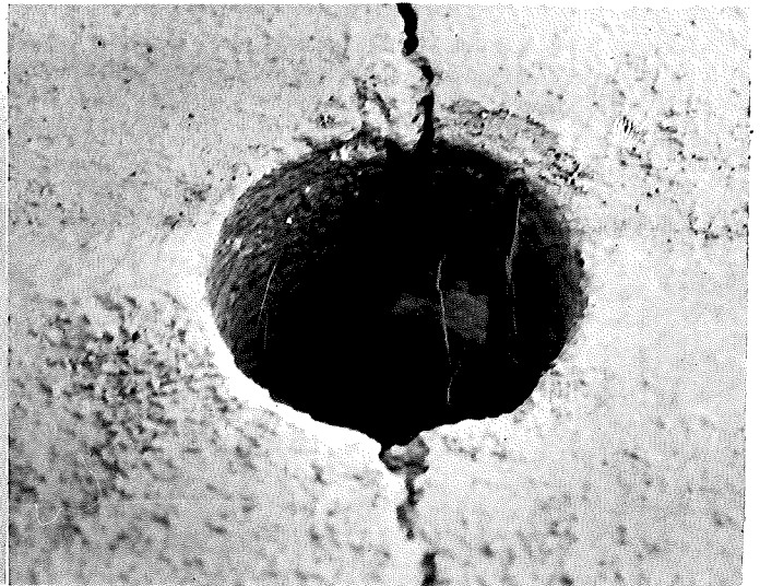
FIGURE 29. VIEW OF CORE HOLE. STATION 159+09 WHERE CORE WAS TAKEN AT CRACK IN CAPPING. DECEMBER 12, 1952.
