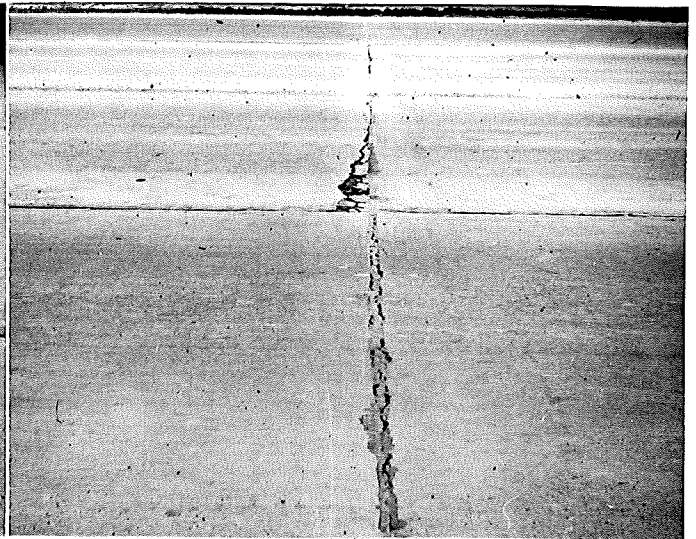
FIGURE 27. JOINT DISINTEGRATION IN AREA WHERE 5 1/2" OF CONCRETE CAPPING WAS PLACED. STATION 112+14 NOVEMBER 19, 1952. 112414
