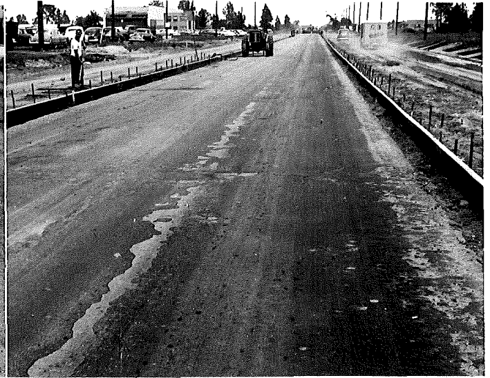
FIGURE 7. VIEW OF THE AE-3 AND SAND TREATMENT AFTER ABOUT A WEEK OF TRAFFIC OVER IT. JUNE 27, 1952.
