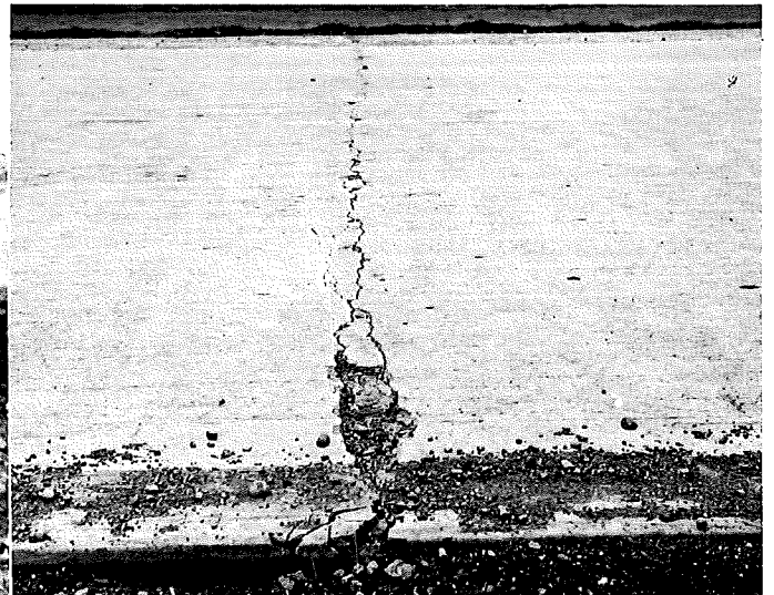
▲ FIGURE 23. APPEARANCE OF CRACK AFTER RECEIVING ABOUT 3 WEEKS OF TRAFFIC. JULY 16, 1952.
