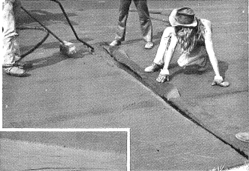
Figure 9. Overlapping two adjacent fabric mats in the direction of laydown; additional binder and brooming was applied manually to minimize pick-up by paving trucks.
