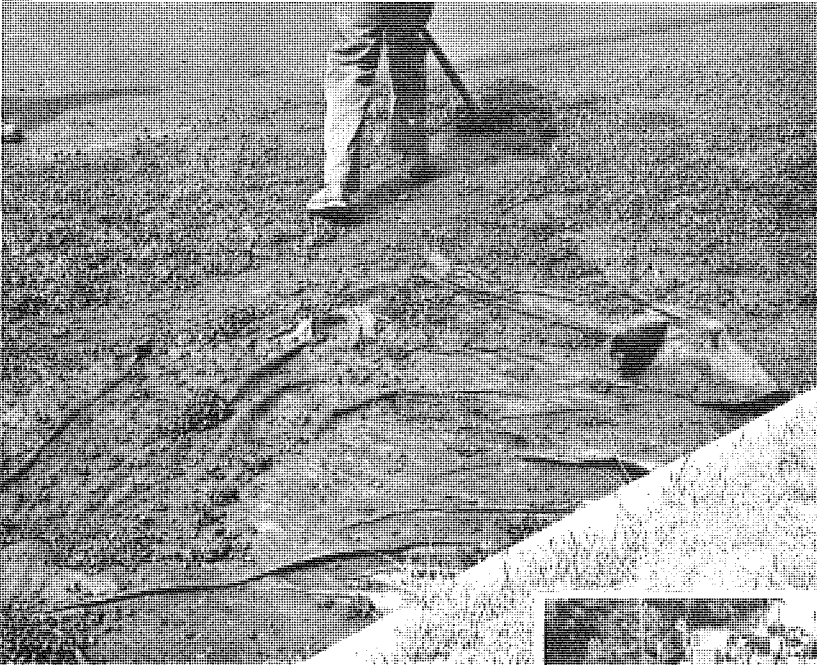
◀ Figure 12. A paving-truck driver inadvertently hit brakes and tore up outside edge of fabric. The damaged section (20-ft long) was cleaned and resurfaced.
