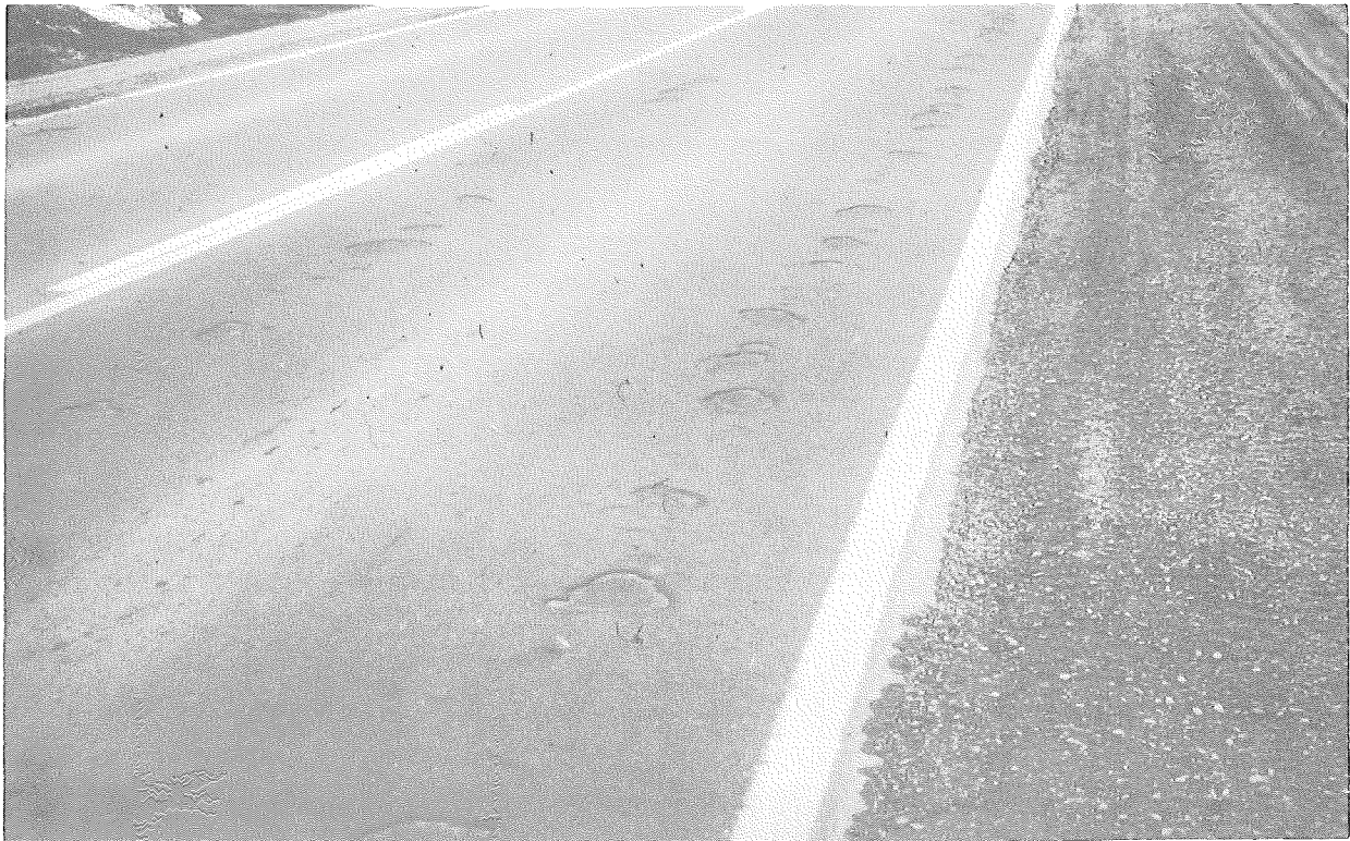
Figure 15. Sand-asphalt surface, 1 year after construction showing delamination.
