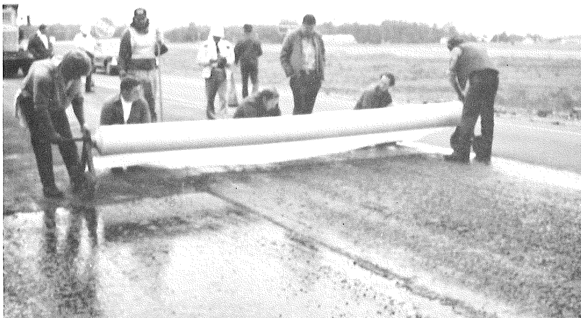
Figure 4. Unrolling, laying down and bonding the first 330-ft roll, 14-3/4 ft width, of Mirafi fabric, required five men and took more than an hour to place the fabric over the asphalt emulsion.
