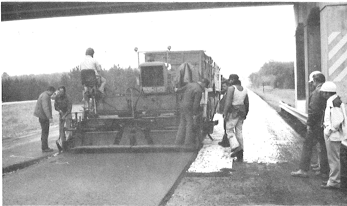
Figure 6. Applying asphaltic concrete overlay to the fabric at a rate of 250 lb/sq yd. The rolling sequence behind the paver required first a 2-ton steel-wheeled roller operating at 3 mph and then another 8 to 12-ton steel-wheeled roller operating also at 3 mph to complete the resurfacing job. Once this lane was compacted and finished, the other lane was ready for the fabric laydown. The two lanes were completed the same day according to plan.
