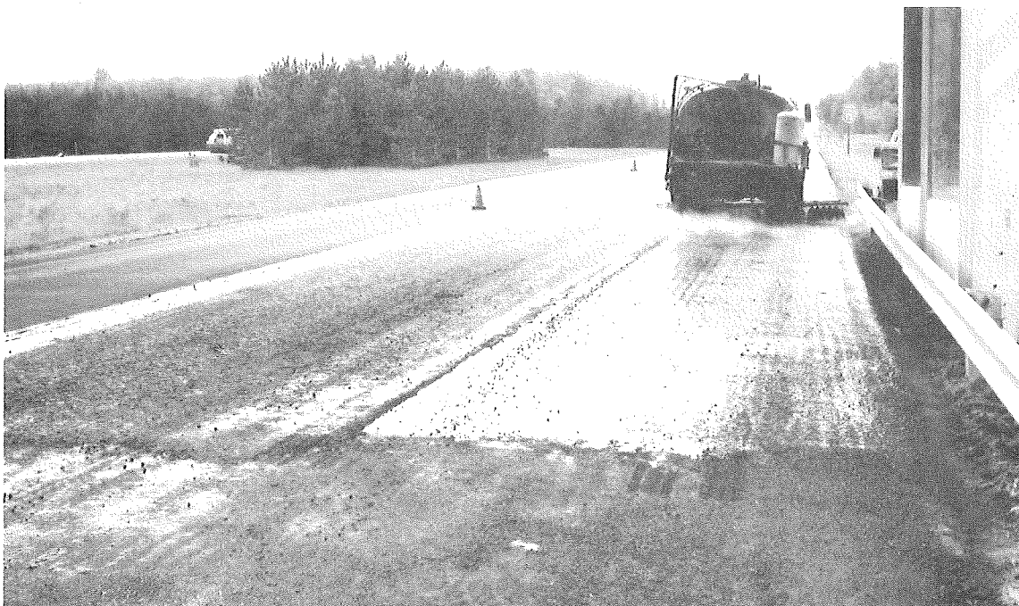
Figure 3. Spraying asphalt emulsion, SS-1h, over the 330-ft traffic lane of the test section. The emulsified asphalt was applied at temperatures over 300 F and at the rate of 0.15 to 0.20 gal/sq yd.
