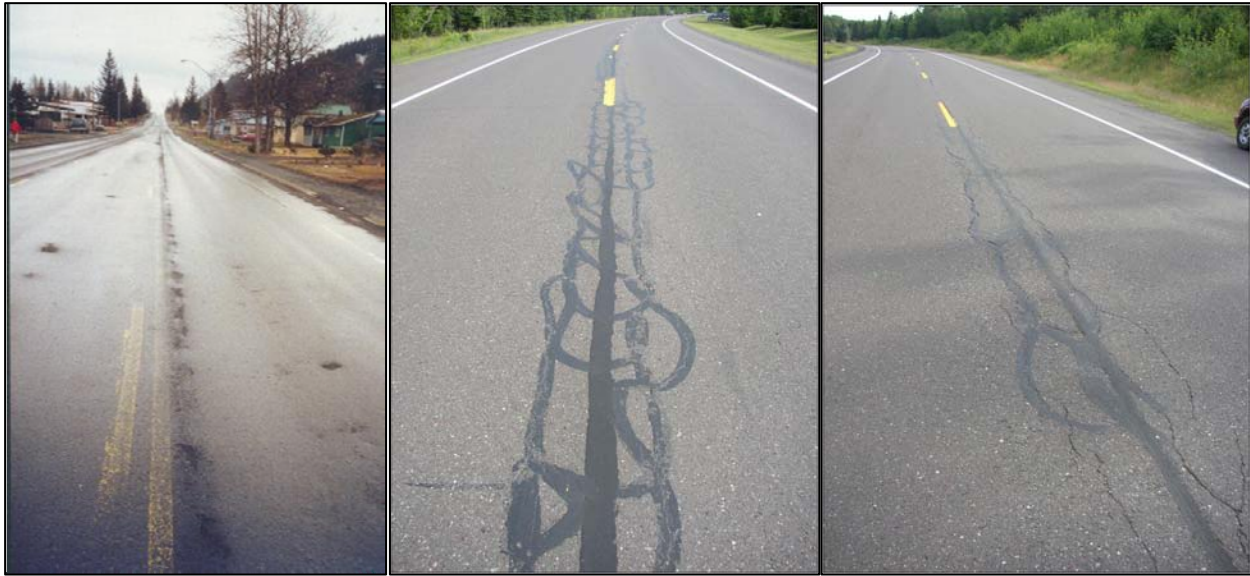
Figure 49. Cracking and Accelerated Deterioration Along Longitudinal Centerline Joints that were Inadequately Constructed
