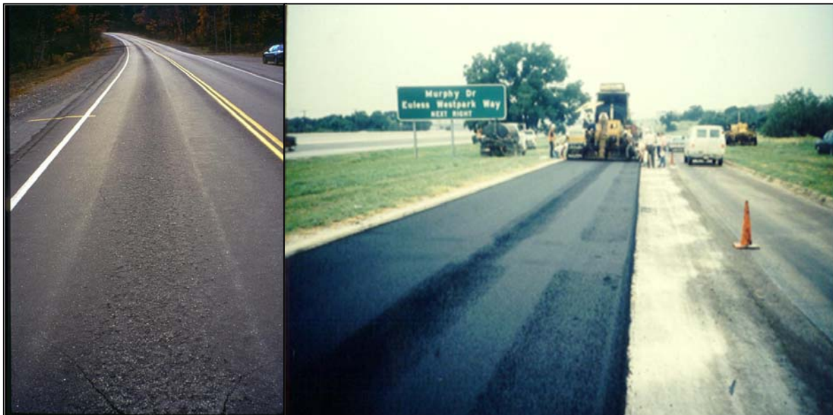
Figure 50. Cracking and Deterioration Along the Center of the Lane where the HMA was Improperly Placed
