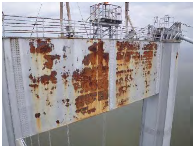
Figure 4.20 - Large area of paint failures on a suspension bridge steel tower strut.
