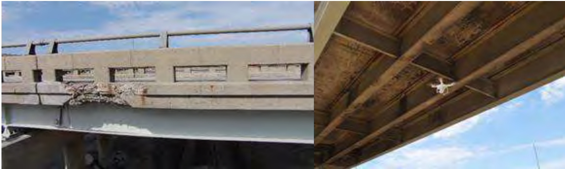
Figure 4.37 - DJI Phantom Vision 2 collected imagery of damage and exposed rebar (left) and girders/beams (right) (Brooks et al. 2015).
