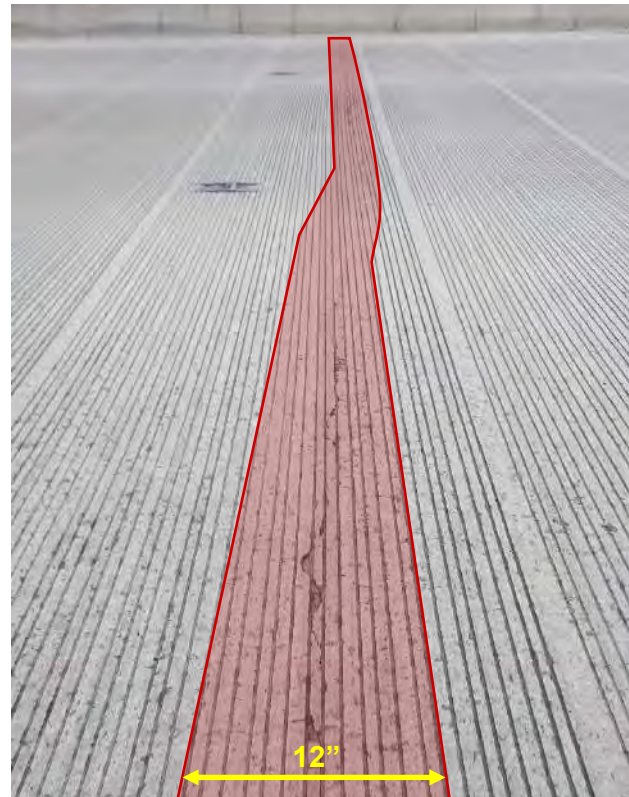
Figure 4.12 - Typical transverse crack in a reinforced concrete deck with 12" wide affected area illustrated.
