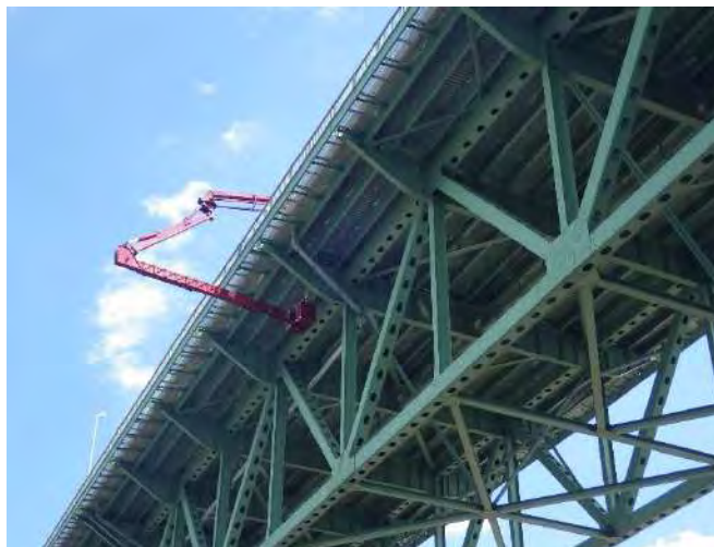
Figure 4.21 - UBIU being used to inspect the Walt Whitman Bridge deck truss approach spans.
