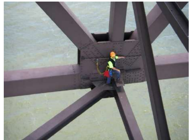
Figure 2.4 - Inspector using permanent hand lines installed along lower chord of the Newburgh-Beacon Bridge.
