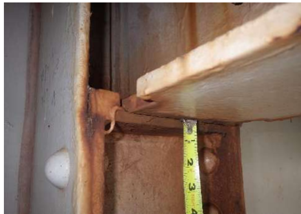
Figure 4.13 - Wear and fretting corrosion occurring at a sliding plate stringer bearing.
