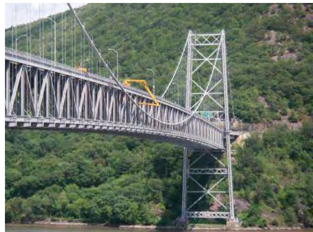
Figure 2.1 - UBIU used to access the floor system and stiffening truss of the main suspension span of the Bear Mountain Bridge.
