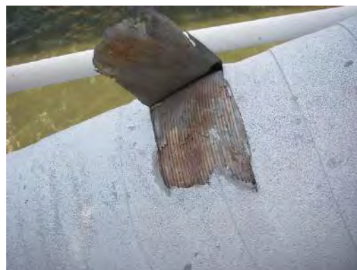
Figure 4.8 - Tear in Cable Protective System material, exposing wrapping wires.
