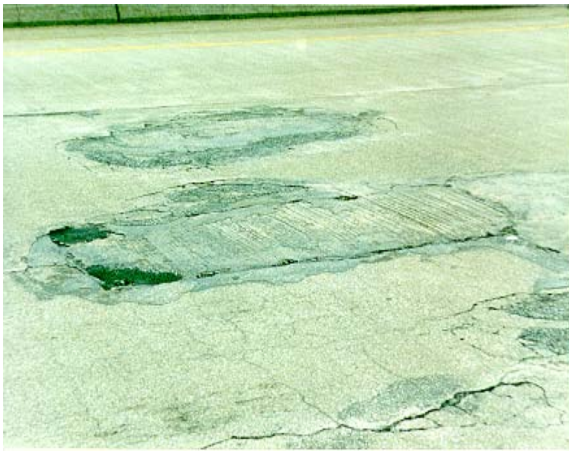
Figure 6 - Repair patch of spalled bridge deck. Map cracking of the deck also shown in the foreground.
