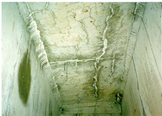
Figure 8 - Transverse and longitudinal cracks and leachate shown on bottom surface of the bridge deck.
