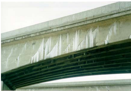
Figure 11 - Shear cracks on beam stem.
