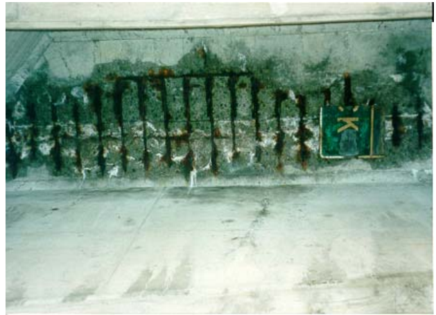
Figure 7 - Delaminated area on bottom surface of the deck. A sign panel was used as a bottom form to repair the hole in the deck.
