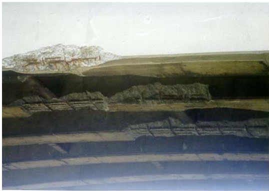
Figure 9 - Large spalls on the beam stem.
