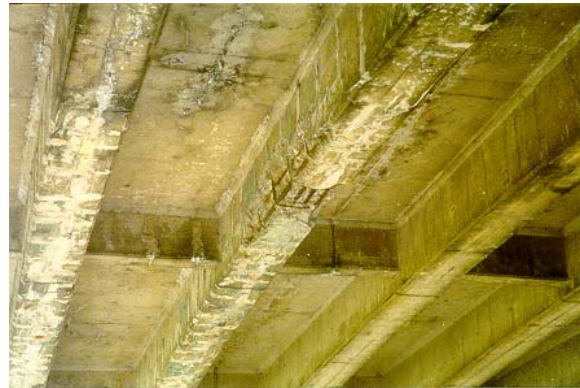
Figure 10 - Flexure cracks on beam stem (epoxy injected).
