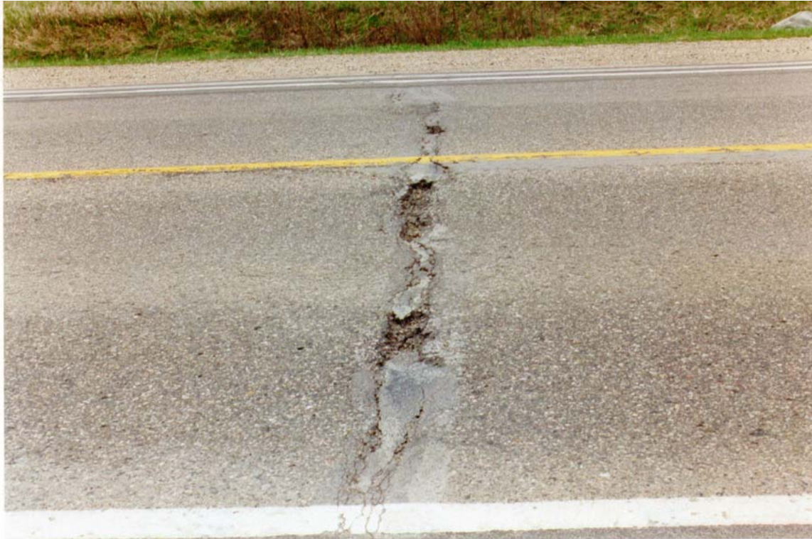
Figure 2 Typical crack with associated distresses.
