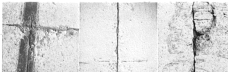
Spalling at center joint
