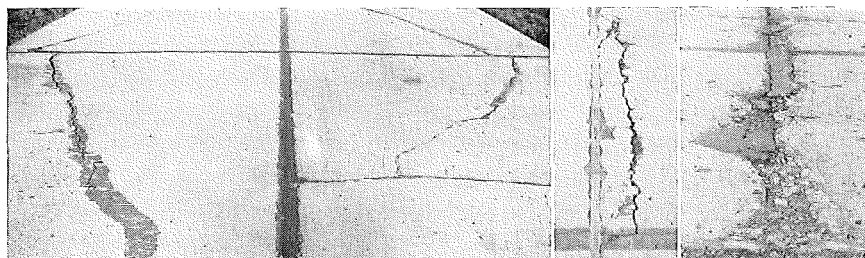
Longitudinal cracking—Infiltration at edges
