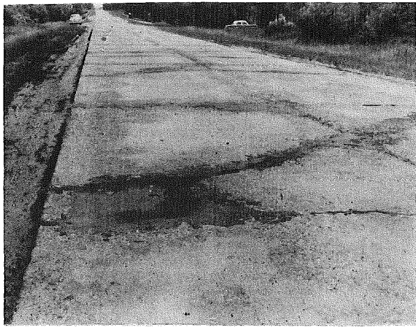
Section 6A Station 94+25 Looking South at Frost Heave Area
