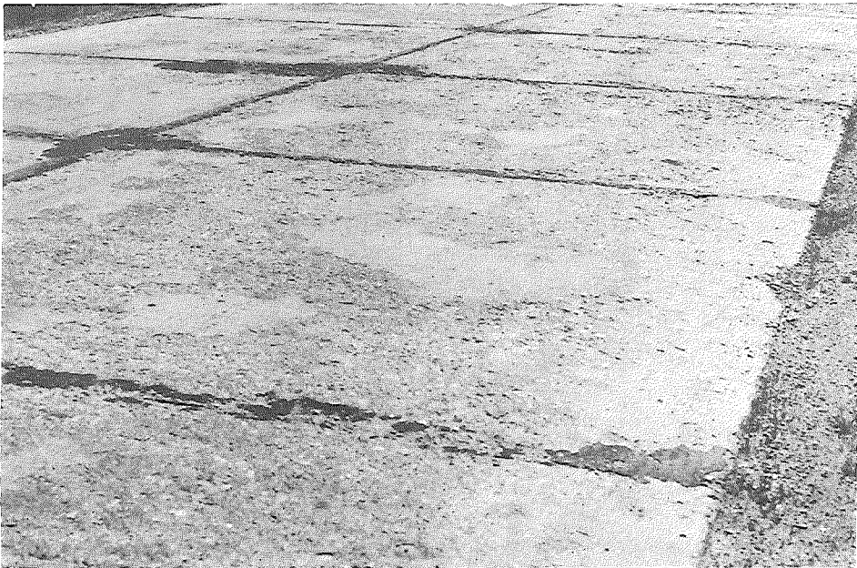
Figure 24. Heavy Scale of Pavement Surface, Section 4E
