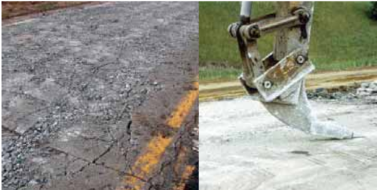
Figure 2-2. Typical concrete pavement break pattern before removal (left) and Rhino horn attachment for use in separating concrete for removal (right) after (ACPA 2009).
