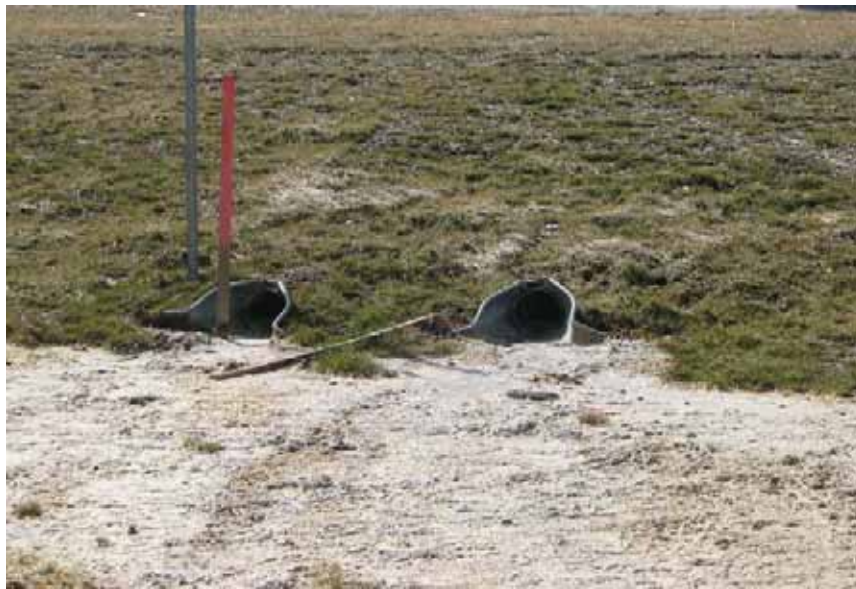
Figure 5-3. I-75 near Bridgeport; Precipitate from high fines crushed concrete OGDC under shoulder.
