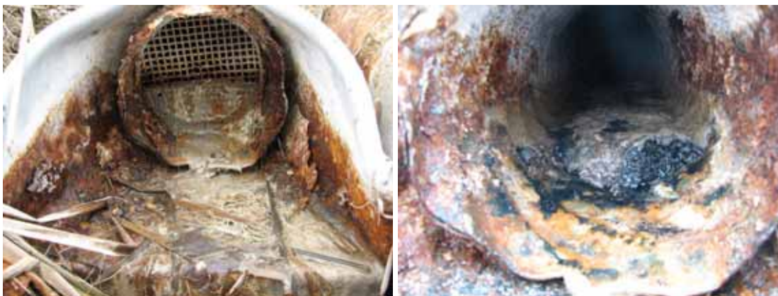
Figure 5-2. I-69 east of Flint; (left) partially plugged rodent screen; (right) blast furnace slag sludge behind screen.
