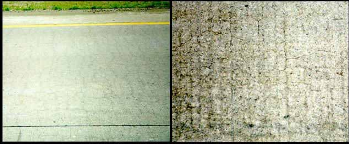
Figure 2-16. Concrete pavement containing RCA as aggregate on I-94 WB, West of Kalamazoo.
