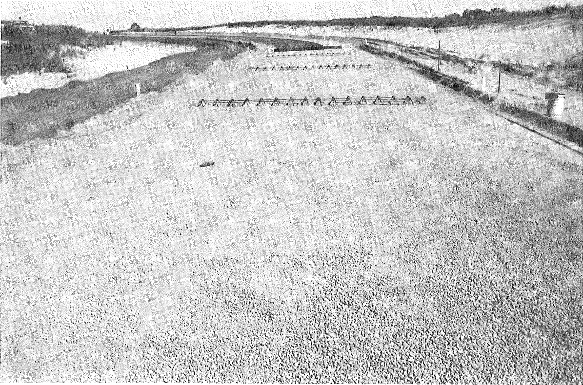
Figure 4. Appearance of slag base after fine grading operations—showing segregation that could restrict lateral drainage to OGDC drains.
