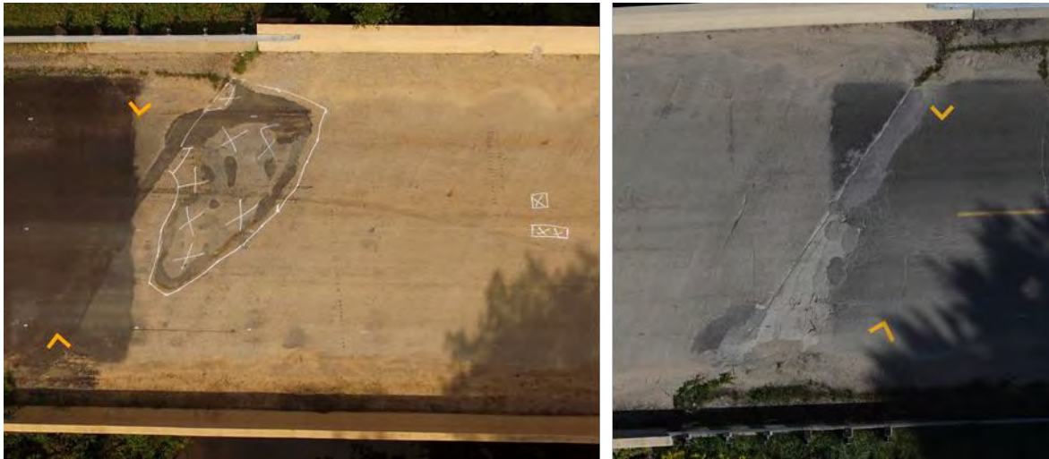
Figure 4: Example digital camera images from the Gordonville Road site: a DJI Phantom 3A image showing surface patching and sounding survey markings (left); a Nikon D810 image showing part of the bridge with distresses at the eastern bridge joint. Both photos have GPS ground control markers visible (yellow chevrons).
