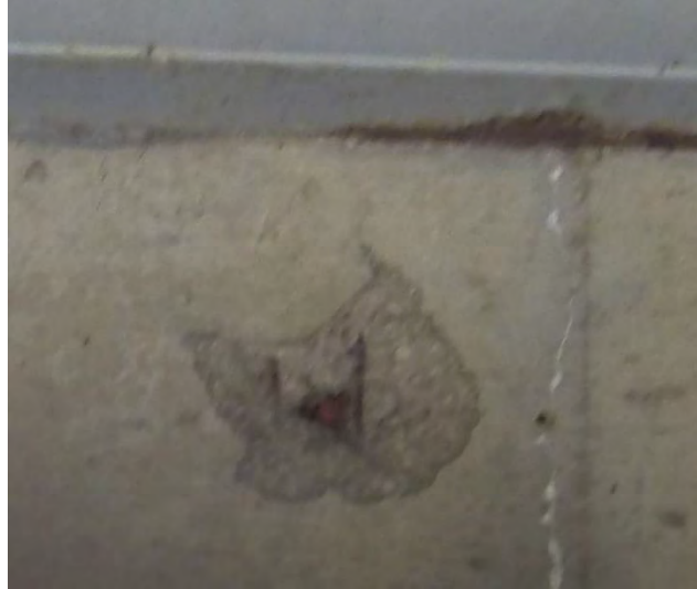
Figure 54: Zoomed-in view of part of the underside GoPro image featuring a spill that was visible using the waterproof UAV, without having to send a person under the bridge.
