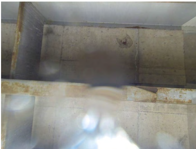
Figure 53: Example photo taken with the top-mounted, upwards facing GoPro while the Splash UAV performed a powered float underneath the test bridge, providing imagery of a spall despite the lens cover being wet.
