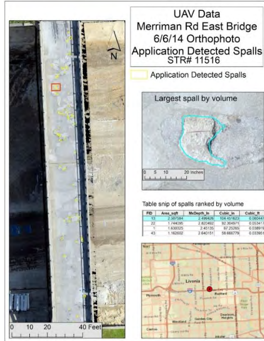
Figure 78: Spall layer of the Merriman bridge with close-up of the largest spall by volume selected from the attribute data.
