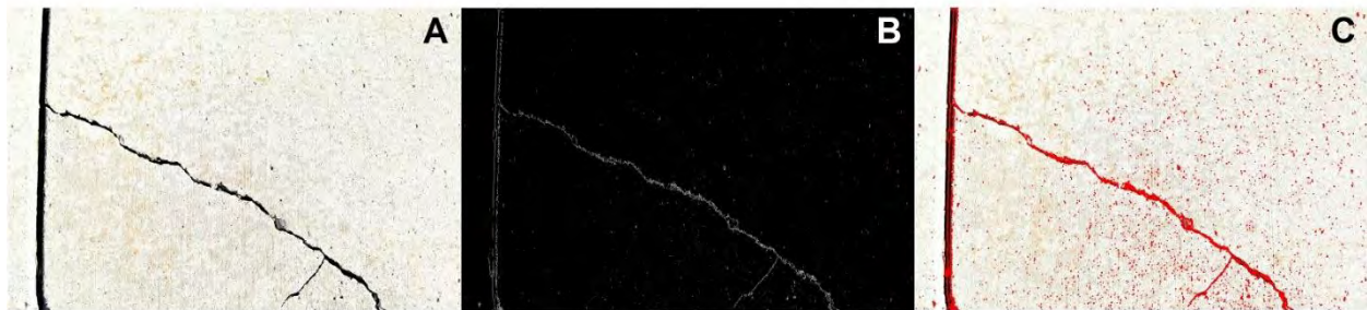
Figure 98: A. The original image of concrete containing cracks. B. Output from Matlab code where white is “detected” crack. C. Final merged product over original image.
