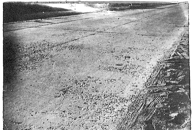
Typical Scaling at Getty Avenue
