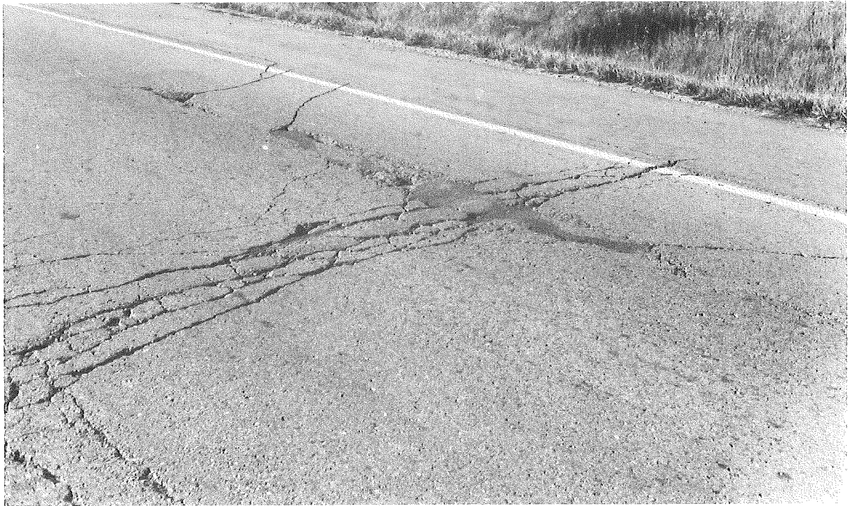
Disintegration of Sulphlex over joint in underlying pavement.
