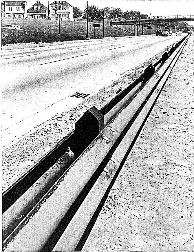
Figure 1. Primed but not field coated railing on West Ford Expressway; installation about 1/2-year old. Dark areas denote rusting.
