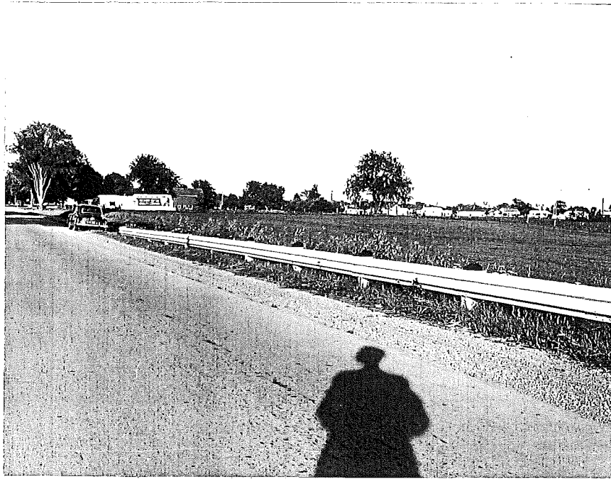
Figure 3. Condition of beam railing on M-50, M-52, west of Tecumseh; installation about four years old. Coating in good condition.
