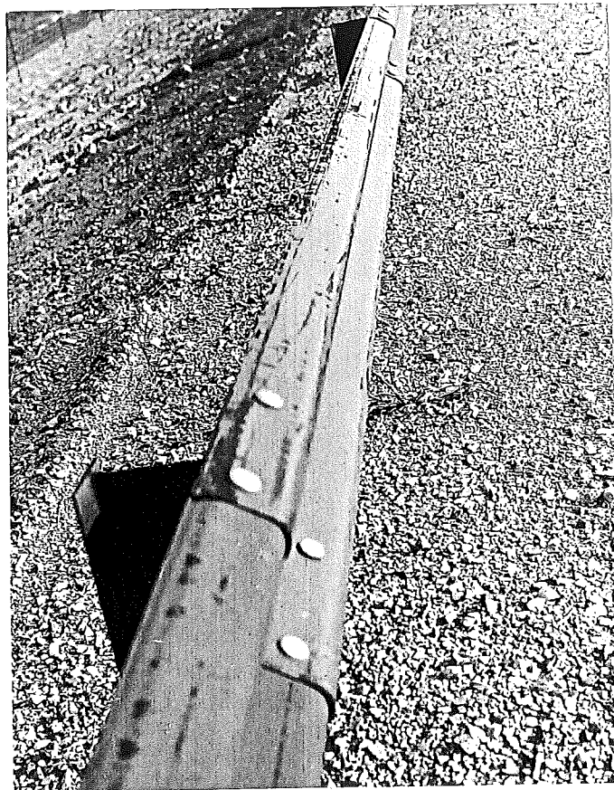
Figure 4. Newly installed factory primed, but not field coated railing on US-127; Station 1056/60. Dark areas denote rusting.
