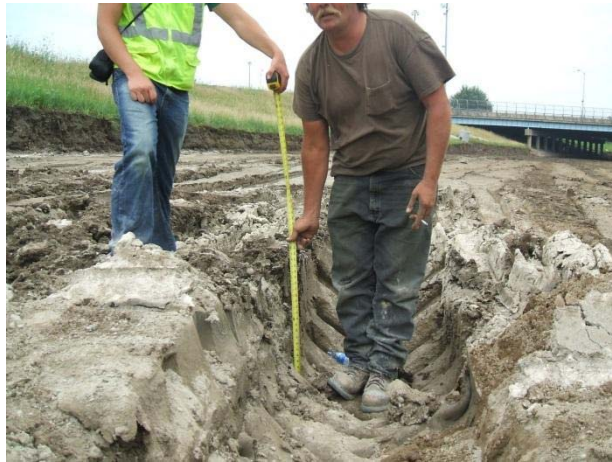
Figure 1.1: Failure of Weak Soil Subgrade under Construction Traffic Loading
