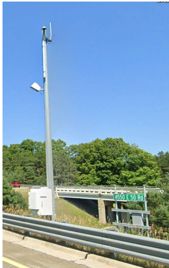
Figure 63. BDWS Non-Invasive Sensor on SB US-131 at E. 50 Road
