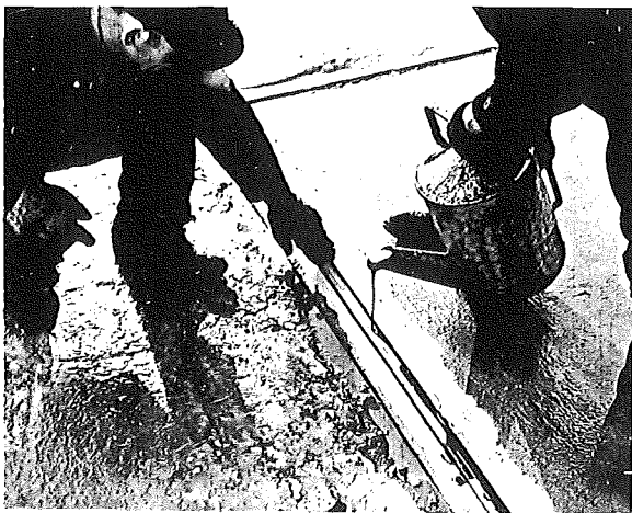
E. ANOTHER METHOD OF CONSTRUCTING DYKES WITH BITUMINOUS MATERIAL AND ONE STRIP OF WOOD
