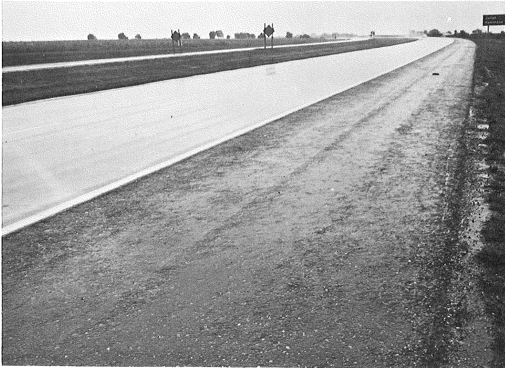
Figure 1. Illinois experimental shoulder installation: non-reinforced portland cement concrete (above) and bituminous aggregate (below).
