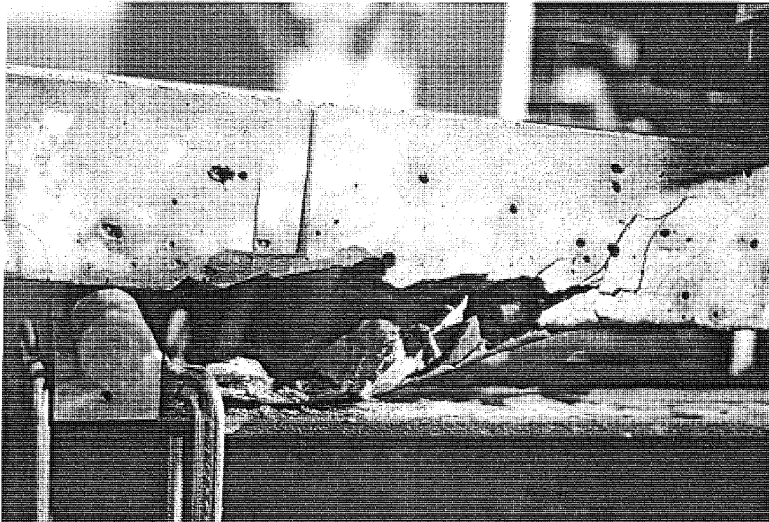
Figure 17. Tonen System. CFRP Peeling-Off Initiated by a Shear Crack
