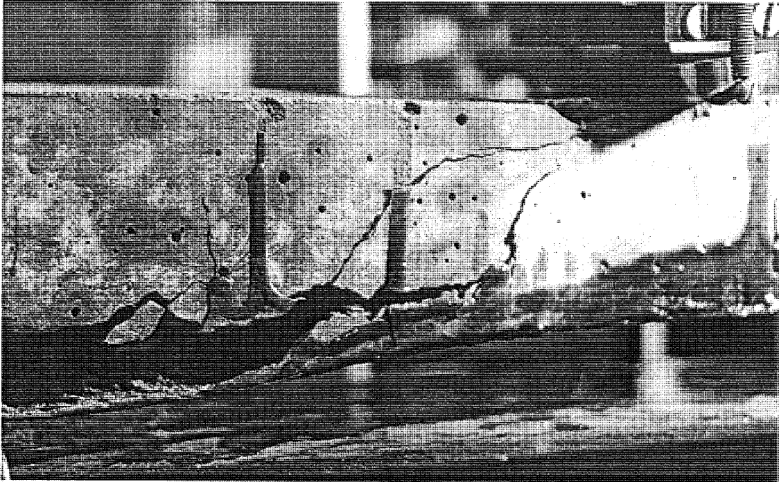
Figure 19. Shear-Delamination Failure of a Specimen with Tonen System
