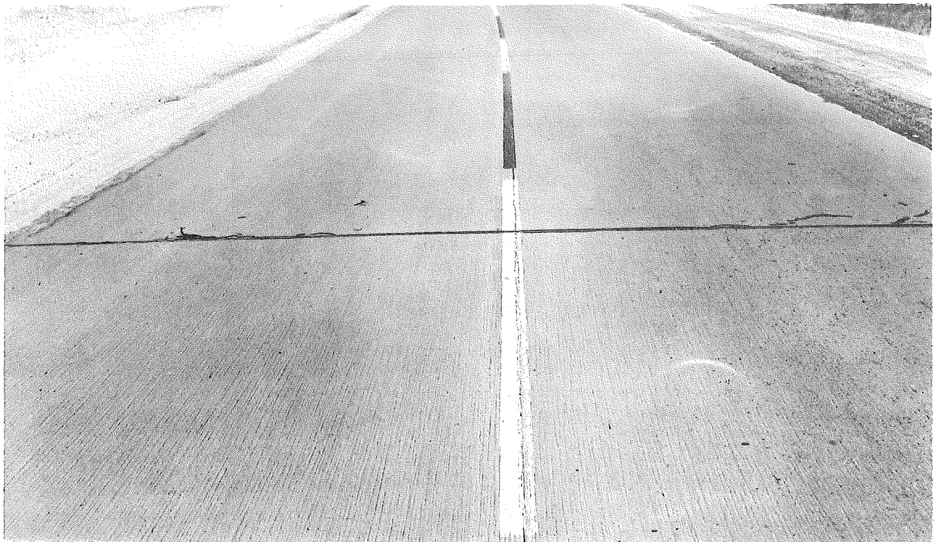
Figure 3. After 14 months of service, this test striping placed at longitudinal centerline shows greatest deterioration over the joint. The area shown was brushed and silicone-pretreated before stripe application.
