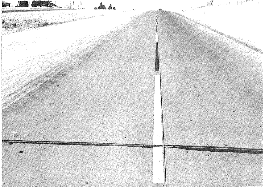
Figure 2. Test initial striping on new concrete (US 23) in good condition after 14 months of service. Area shown is standard striping that received neither brushing nor pretreating before application.
