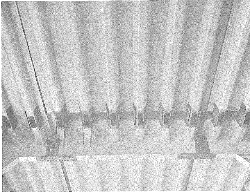
View of bolted connections in the stiffening ribs and floor beams of south span.
