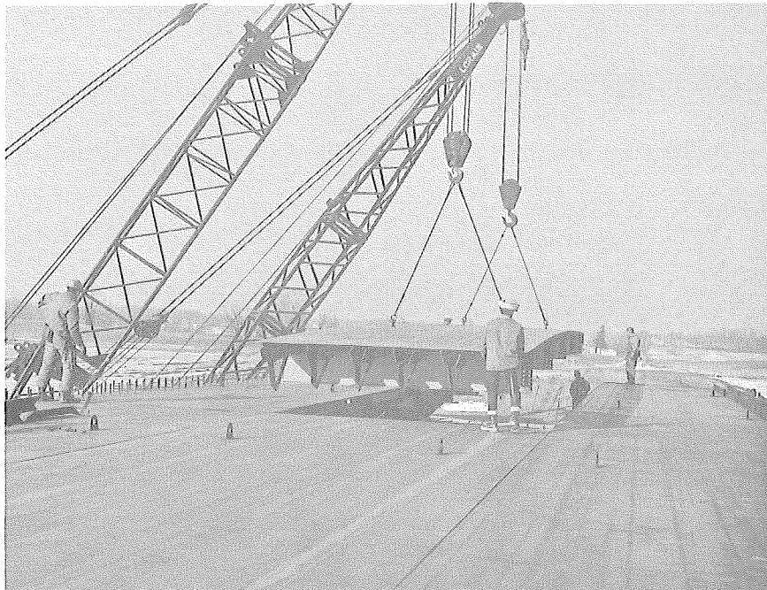
View of positioning the interior deck section in the north span. This was the last deck section to be placed.
