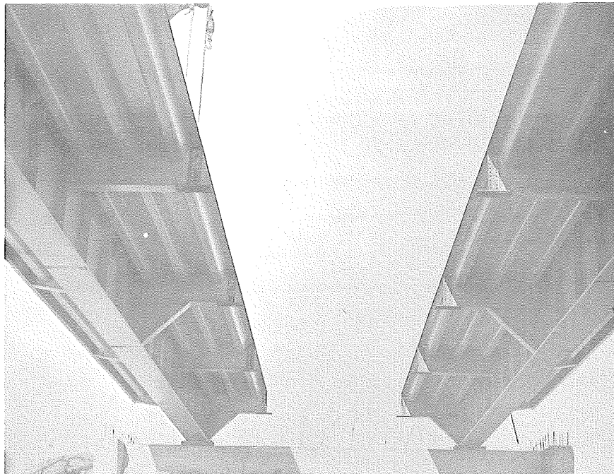
View of the north fascia sections with the splice plates set to receive the center deck section.
