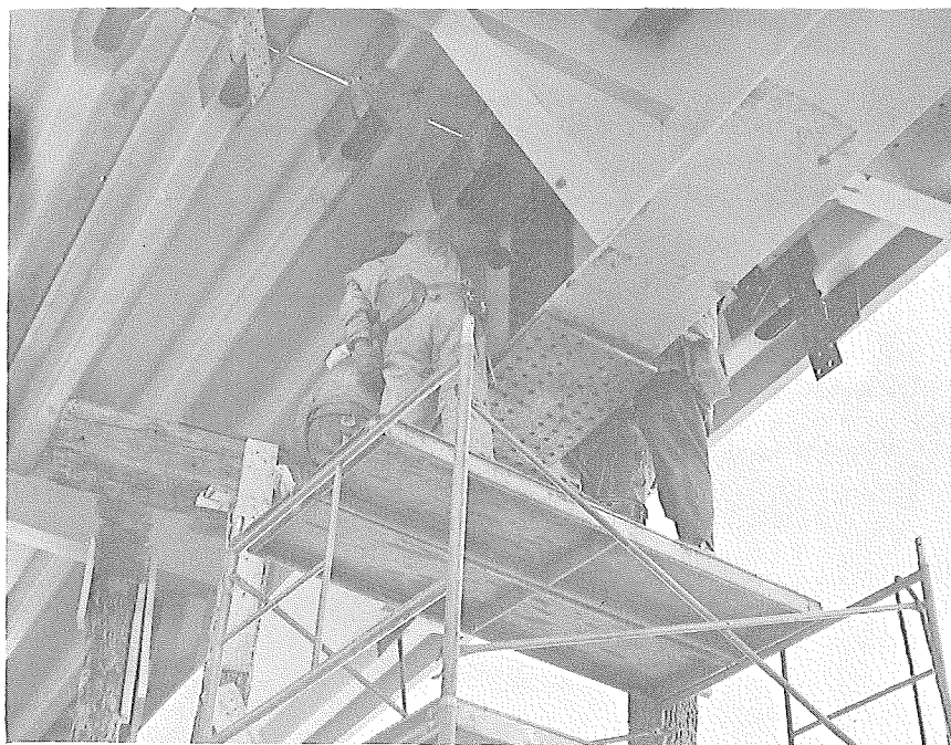
Bolting the field connection in the web of the west girder section of the north span.
