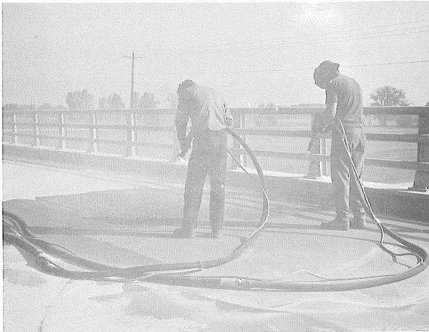
Sandblasting the steel deck plate in preparation for the epoxy primer and mortar.
