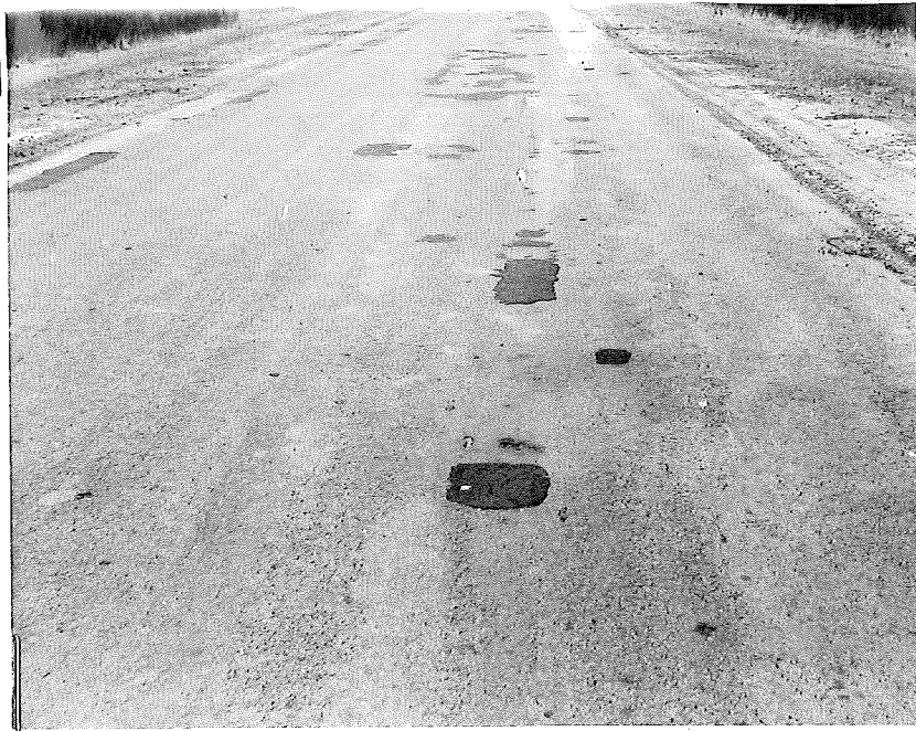
Figure 3. View looking east from Station 30+00 showing recent patching where seal coat has failed.
