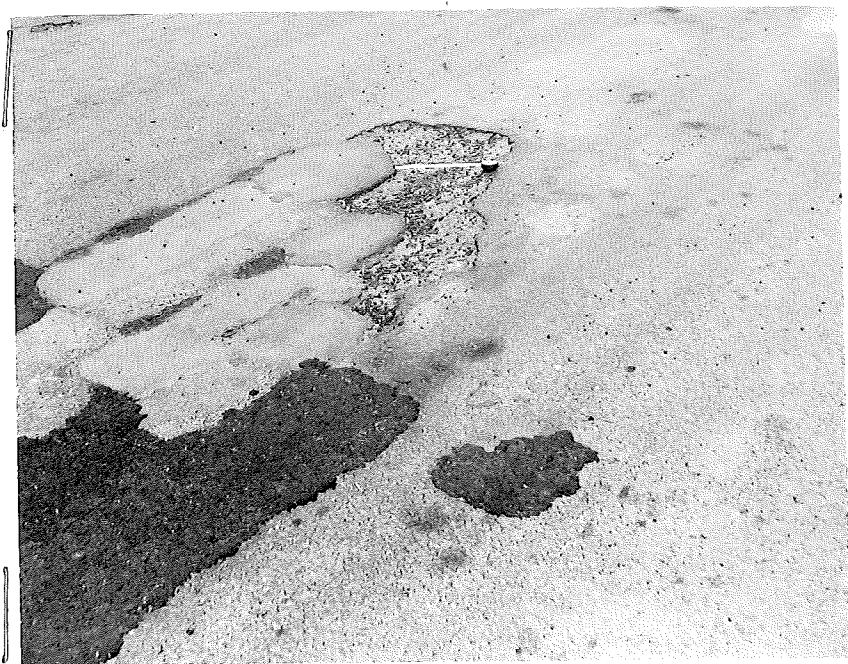
Figure 8. Break in seal coat at Station 45+00 showing progressive breaking of the seal coat and subsequent deterioration of base course.
