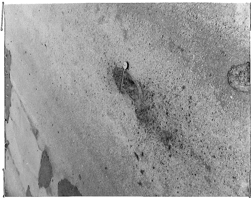
Figure 7. Chuck-hole showing deficiency in bituminous binder. The material could be picked out as easily as the unstabilized soil on the shoulder. Station 45+00.
