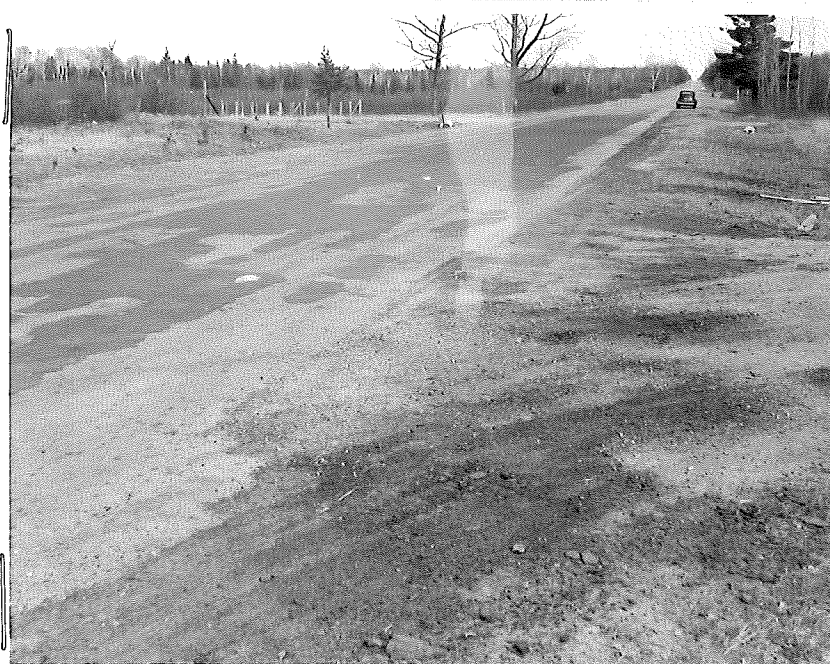
Figure 4. View looking east from Station 34+50 showing area of maximum deterioration which had been patched one week before the picture was taken.
