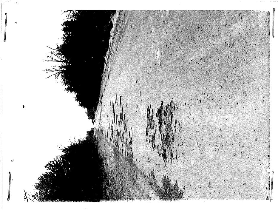
Figure 11. Same type of break in seal coat and rutting of base as shown in Figure 10, also along north lane. Stabilized base material is soft and evidently was poorly mixed. Station 76+50 to Station 79+60.
