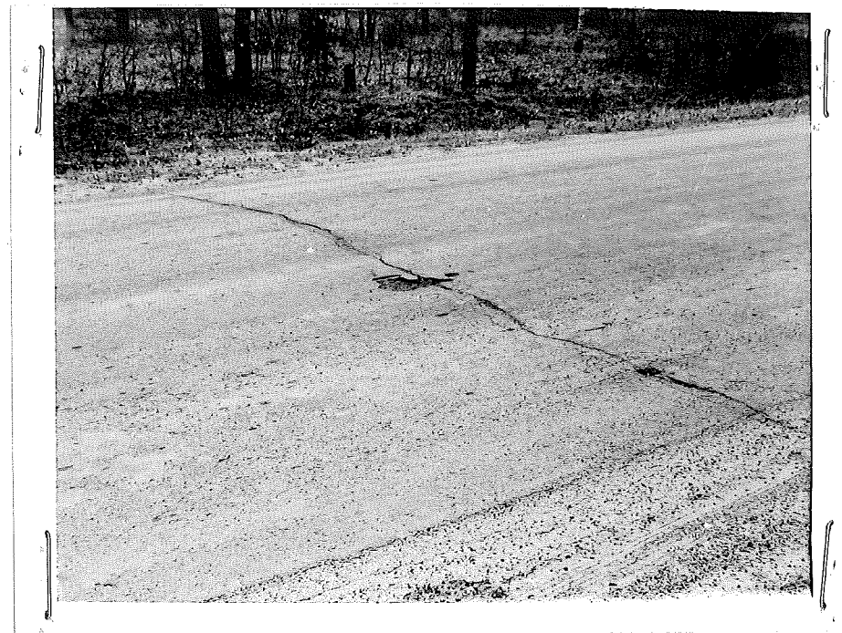
Figure 12. Transverse crack between the AE-7 and the T-3 sections. Note the seal coat beginning to peel off at the crack in center of roadway. Station 80+00.
