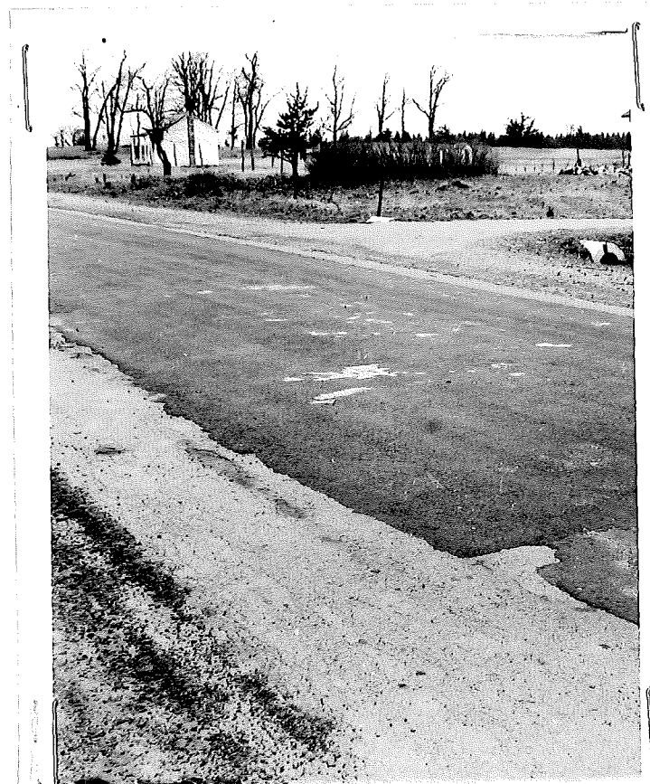
Figure 6. Close-up of large patch in figure 4 showing bleeding (light areas) on new patch.
