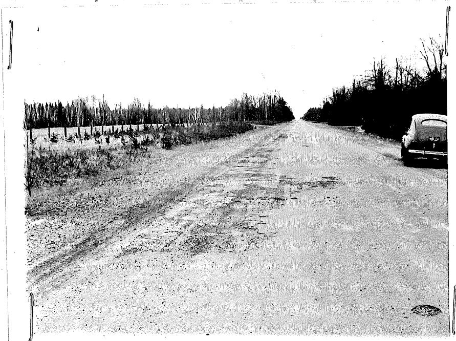
Figure 10. View of large break in seal coat along north lane between Station 57+90 and Station 68+00. Stabilized base possessed very little cohesiveness. Picture taken from Station 68+00. This type of break extended to approximately Station 79+00 which is near the end of the AE-7 bituminous mix section. The AE-7 section ends at Station 80+00.
