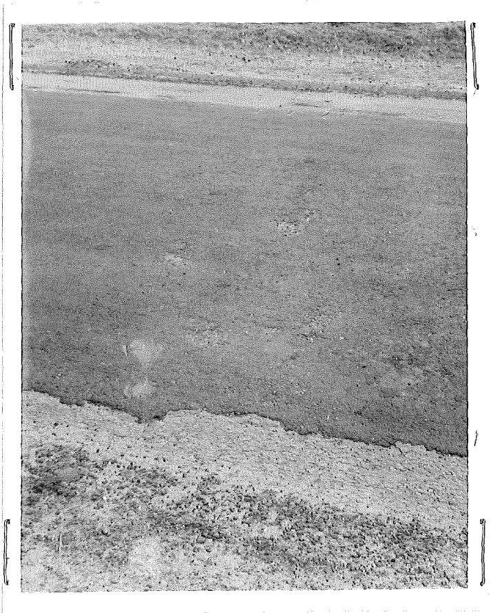
Figure 5. Close-up of large patch in figure 4 showing new patch beginning to peel off of old surface due to improper bond and insufficient thickness of patch. Station 42+00.
