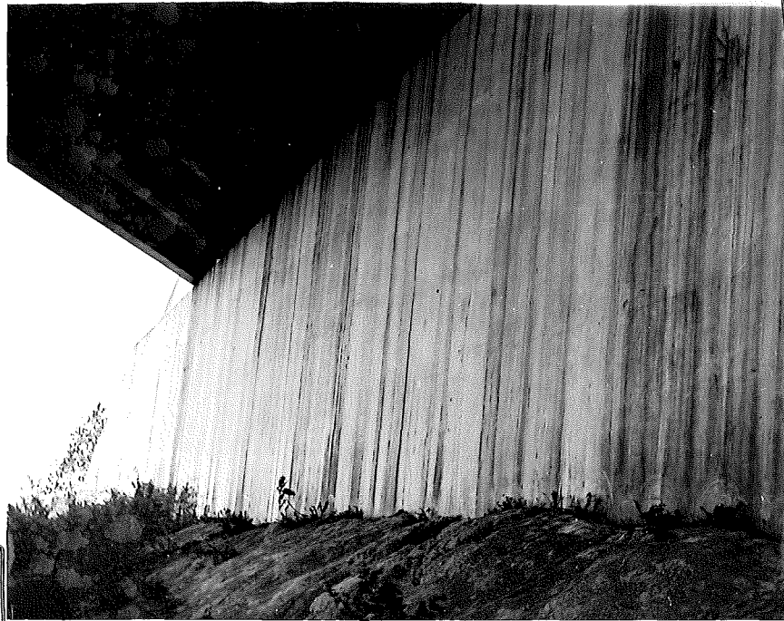
Figure 9. Staining of paint due to surface water. Landing airport overpass.
