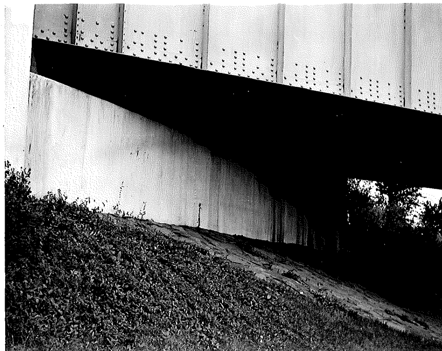
Figure 10. Staining due to surface water. Howell underpass.
