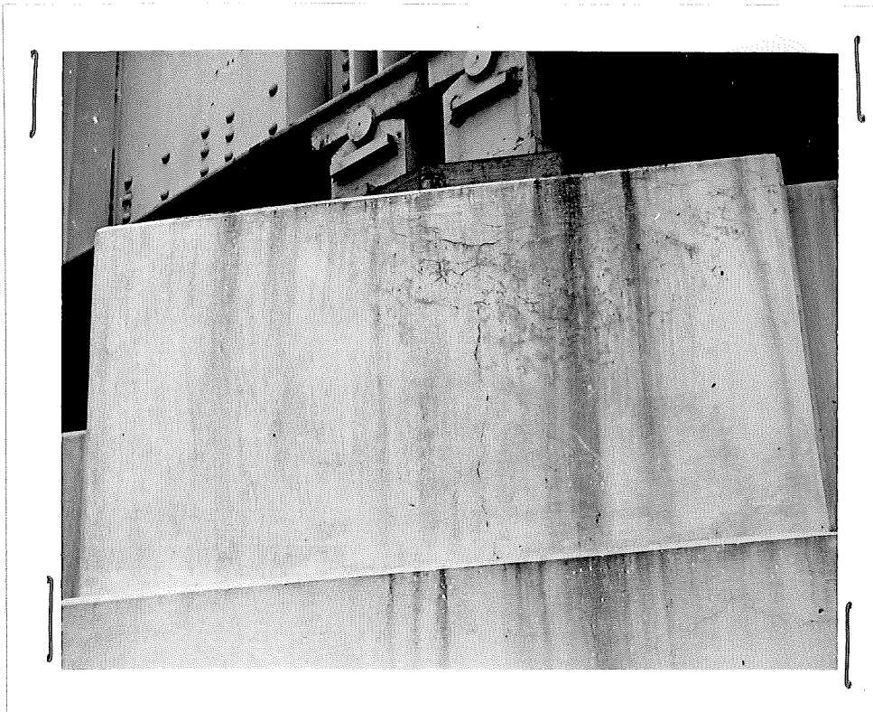
Figure 7. Another example of accelerated weathering of concrete indicated by network of cracks near the top of the wall, US 16 east of Howell.
