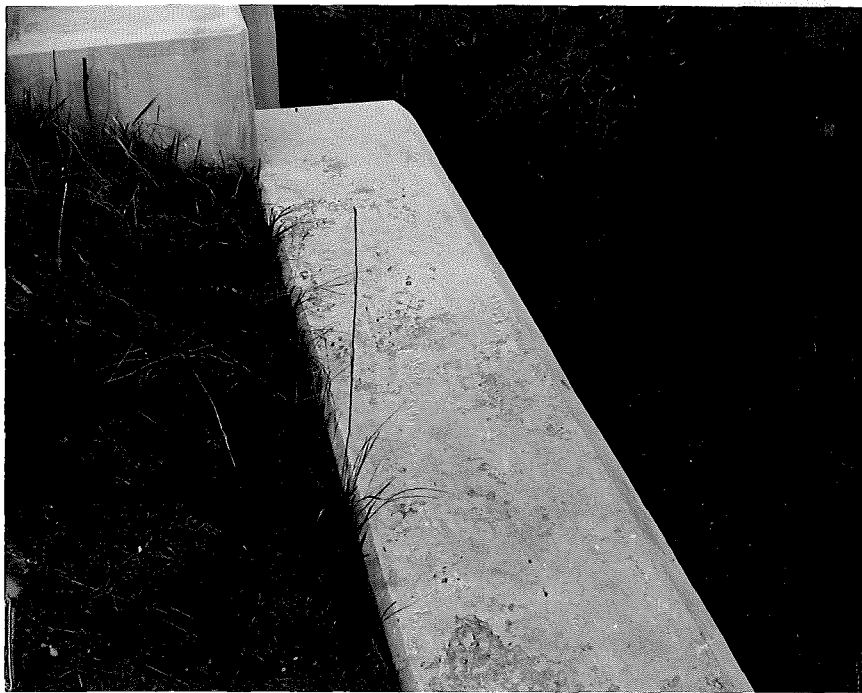
Figure 1. Top of culver wall at Charlotte painted with oil paint in 1944. Note extensive flaking of original coating.
