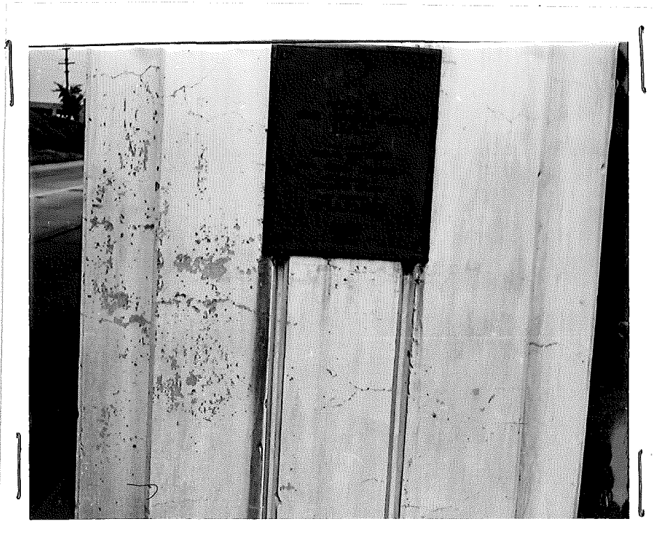
Figure 5. Chipping and sealing of portland cement paint film on underpass east of Howell on US 16. Painted in 1944.
