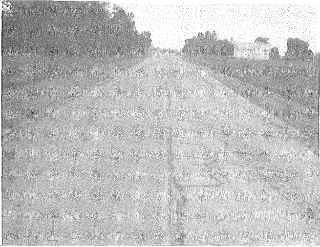
Photo 1. M 57 Before. Transverse thermal cracking, some alligator cracking in wheel-paths, and edge of pavement cracking all in evidence.
