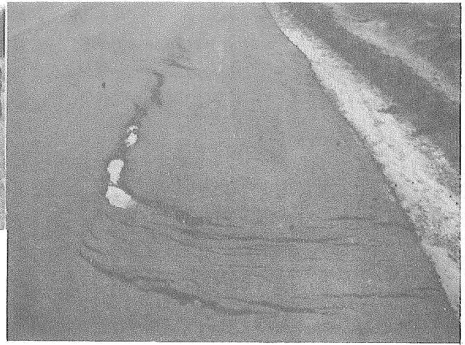
Photo 13. Valuable lesson--this is what can happen when not all of the old material is removed. The resultant is a poor bond and slippage of thin pavement. This area was removed, repaired, and resurfaced with one more course.
