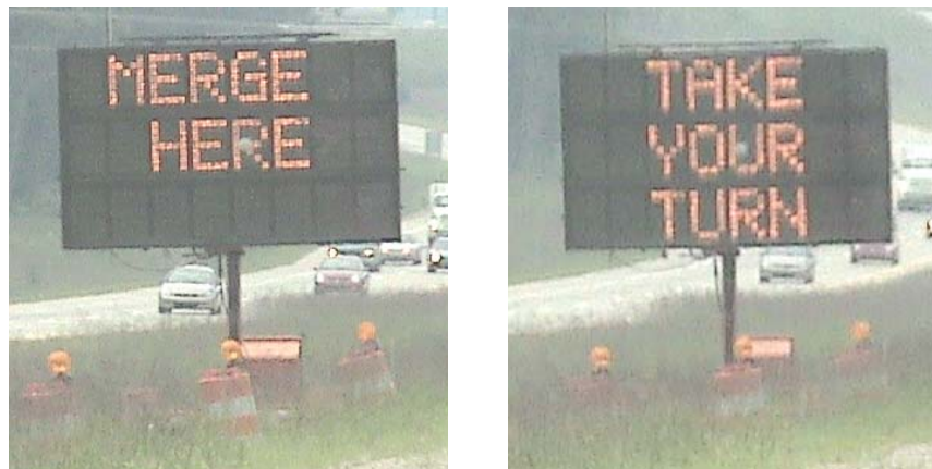
Figure 11. PCMSs Used in the Advance Warning Area
