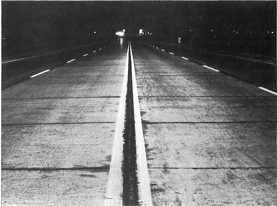
Figure 5. Four-lane undivided concrete pavement at night, showing yellow centerlines and black-white lane lines.
