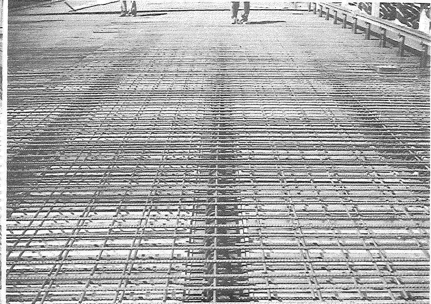
▲ Figure 5. Stay-in-place corrugated metal forms (top left) and deck reinforcement with spiral shear developers (top right).
